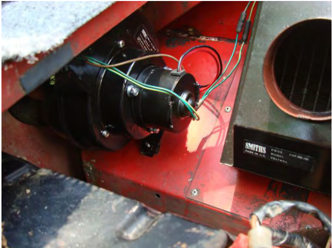
Figure 10. Snail box and fan motor and squirrel cage assembly reinstalled.
