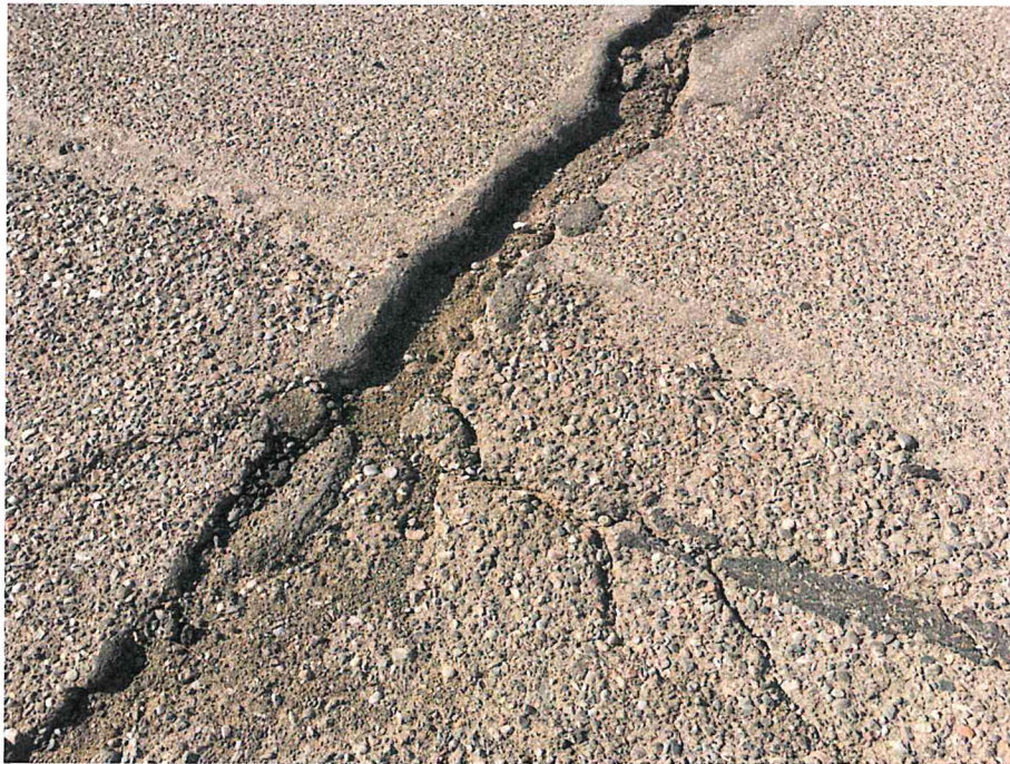
14 th Avenue: Pavement Separation
