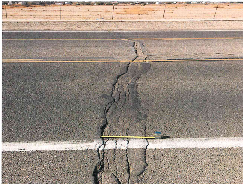
14 th Avenue: Pavement separation
