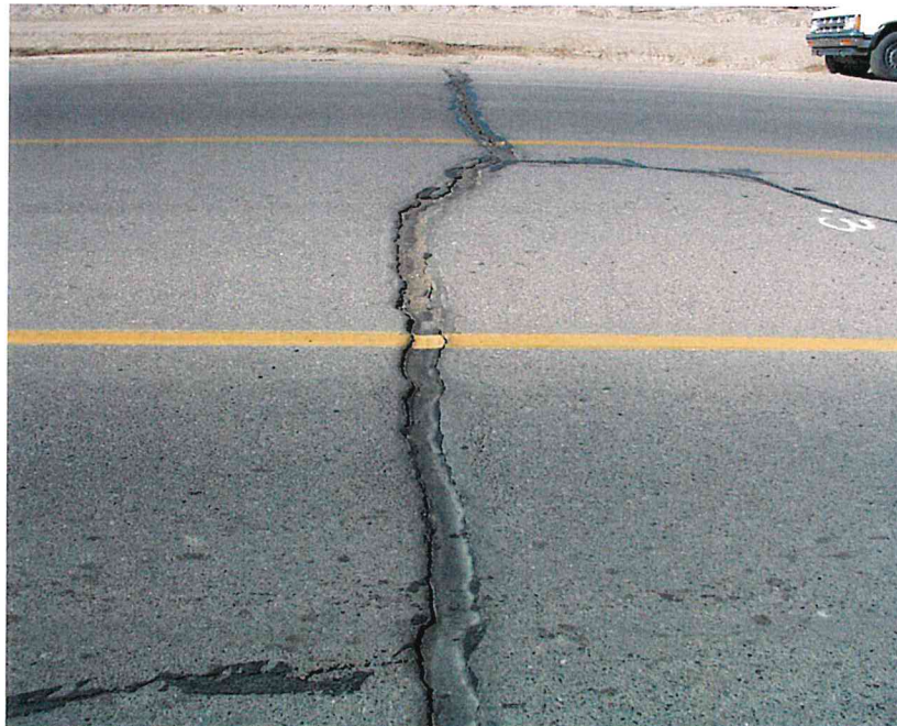
14 th Avenue: Pavement separation
