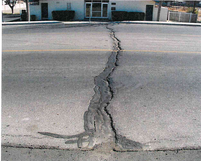
14 th Avenue: Pavement separation
