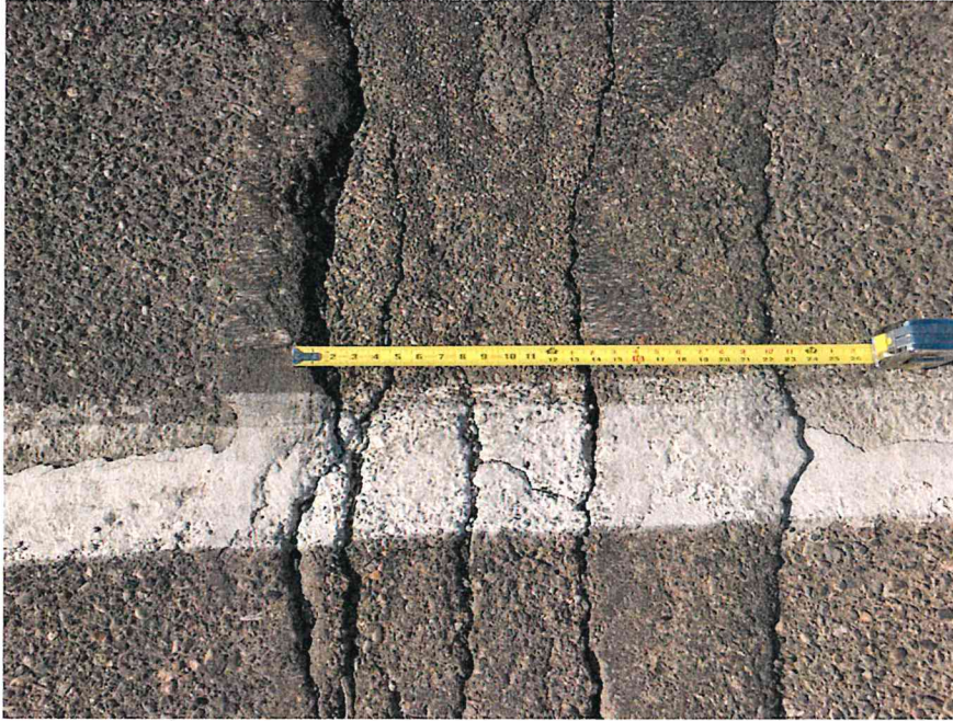
14 th Avenue: Pavement separation 22"
