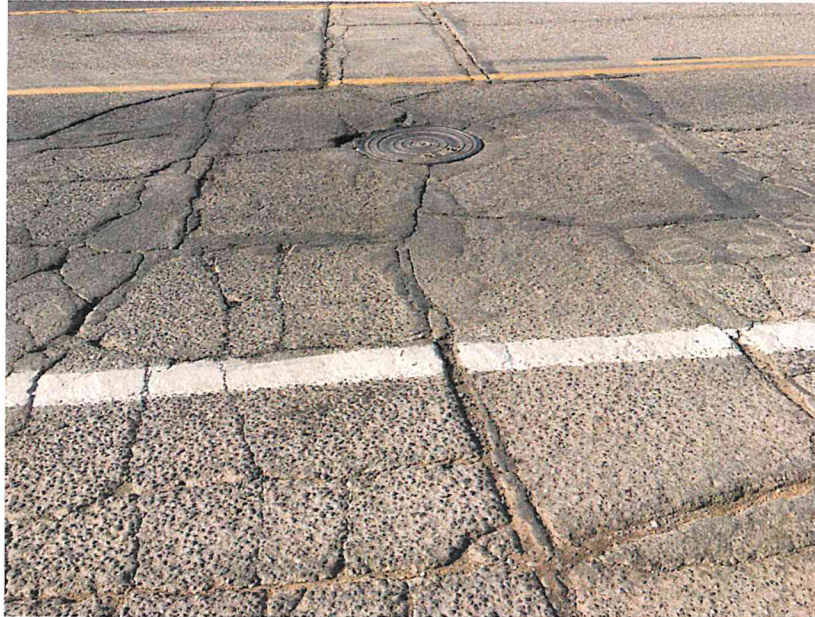
14 th Avenue: East Side, Looking West Deteriorating Pavement
