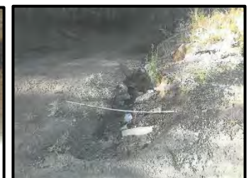
Erosion at the NW
