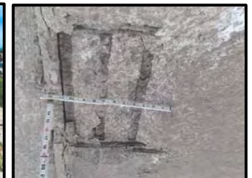
Large Spall in Soffit – Exposing Rebar
