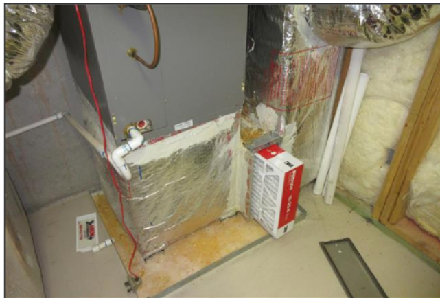
6.0 Item 4(Picture) heat pump
