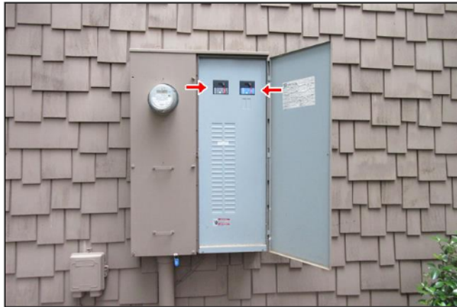
7.3 Item 1(Picture) main disconnect
