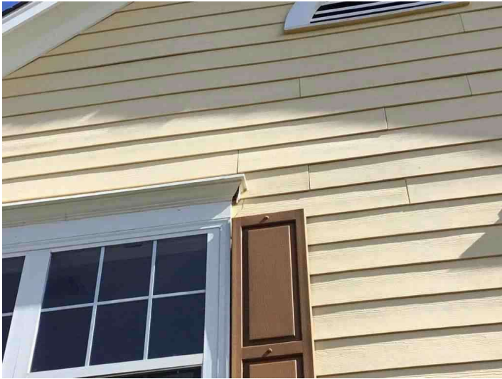
Rotting trim Front window
