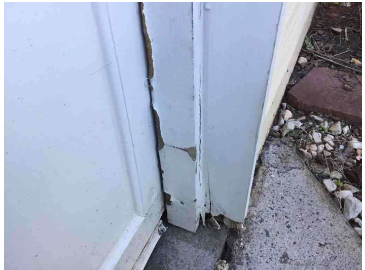
exposed/rotting Garage trim
