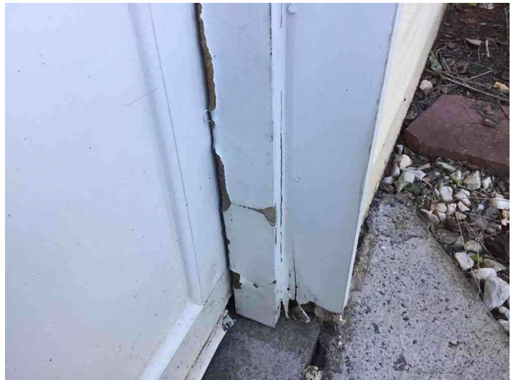
exposed/rotting Garage trim
