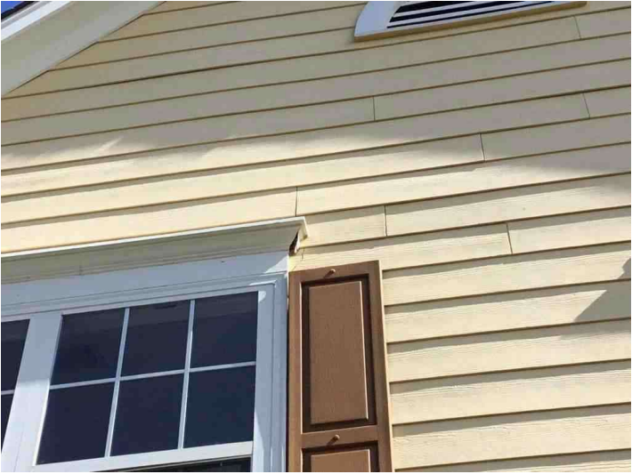
Rotting trim Front window
