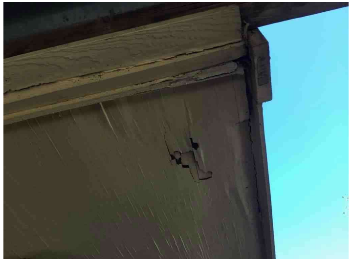
Fireplace soffit rotting
