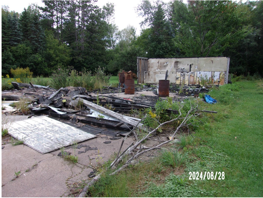
Debris from garage fire from a few years ago not cleaned up.
