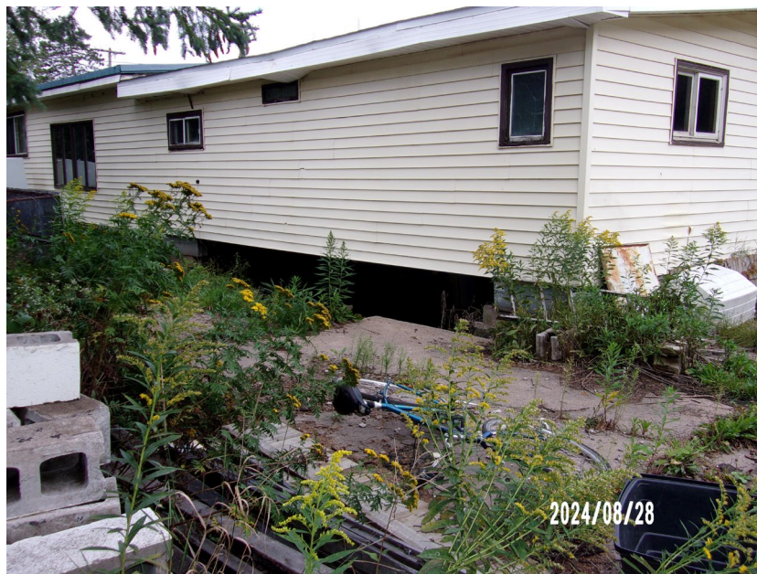
The South foundation wall has collapsed.
