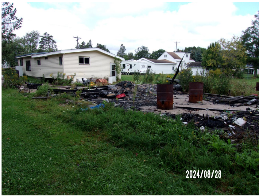
Debris from garage fire from a few years ago not cleaned up.
