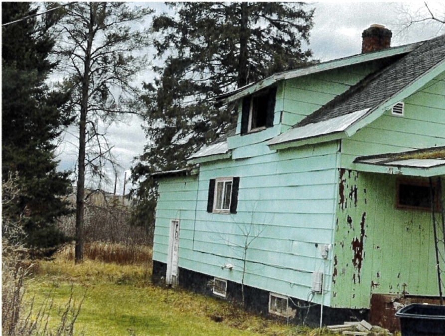
Window missing, fascia falling off on East side of house.
