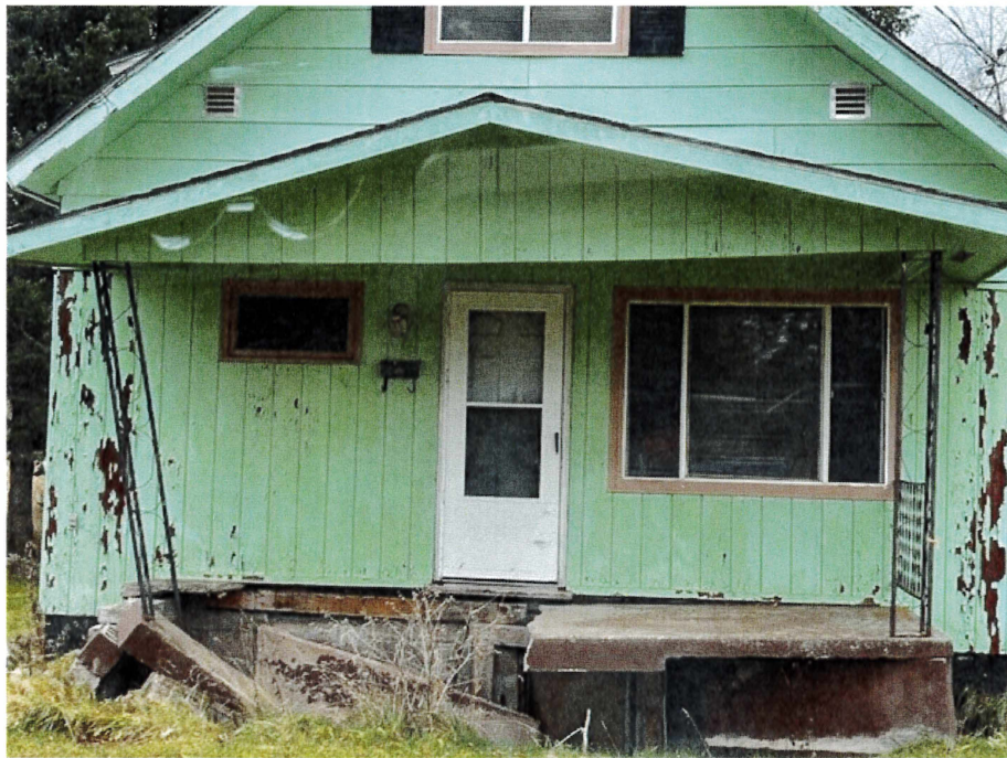
Front porch is falling in and roof support is leaning and non-supportive.
