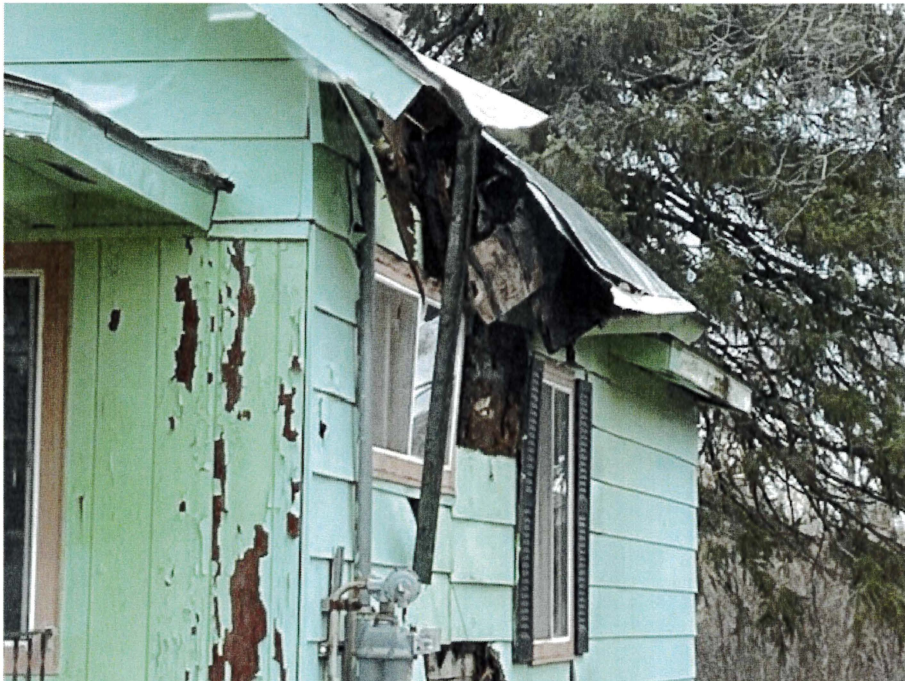
West side eave rotted and falling off.
