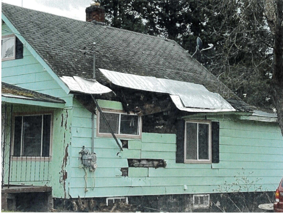
West side of roof and wall deteriorating.
