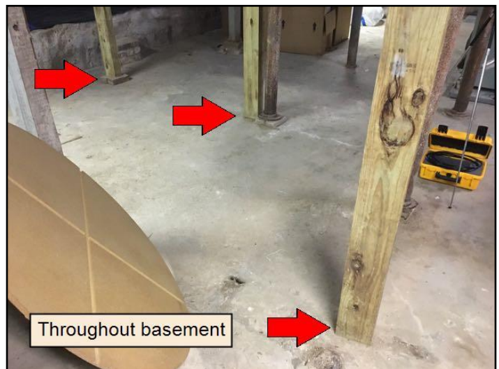
29. Poorly secured at top or bottom Task:...
