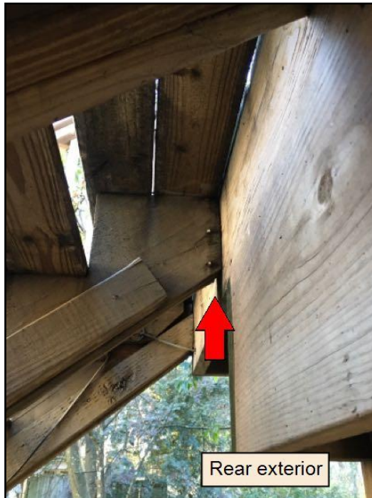
18. Weak/inadequate connections Task:...
