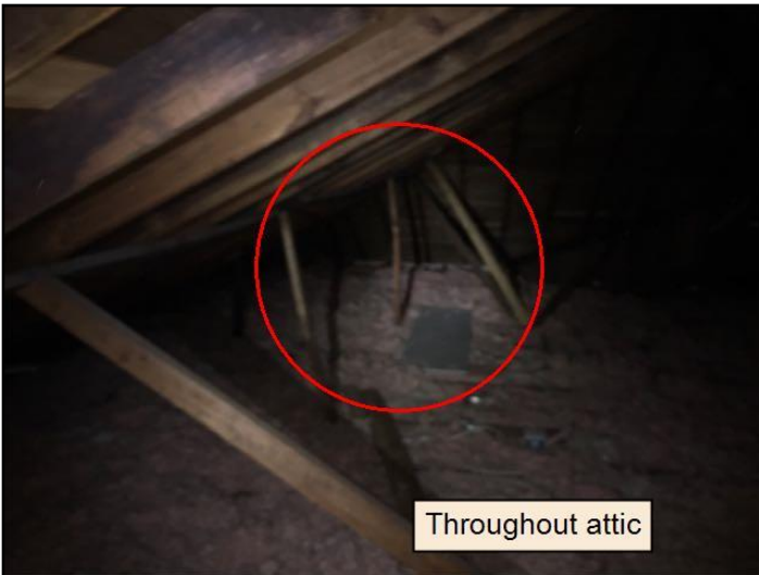
36. Purling Bracing Sagging/Damaged Location:...
