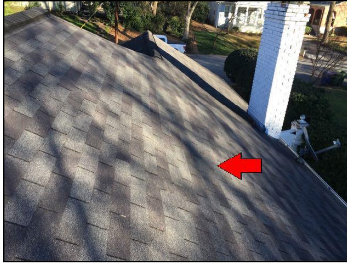
38. Deflection or uneven roof sheathing
