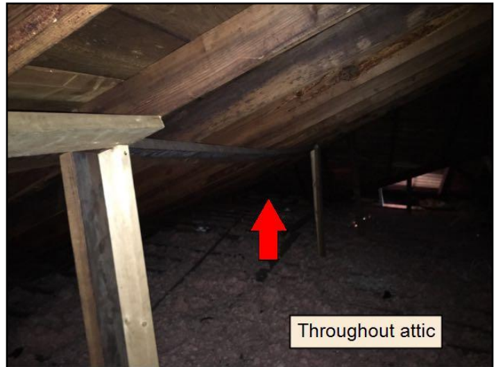
35. Purling Bracing Sagging/Damaged Location:...
