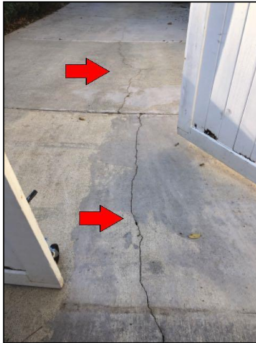
20. Cracked or Damaged Surfaces Task: Repair a...
