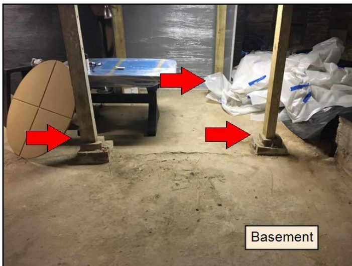
28. Poorly secured at top or bottom Task:...
