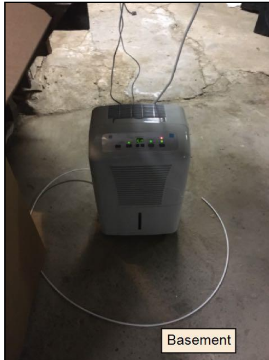
89. Dehumidifier in basement
