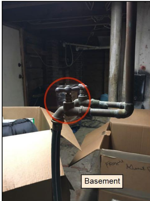
62. Drip/Leak Task: Repair Time:...
