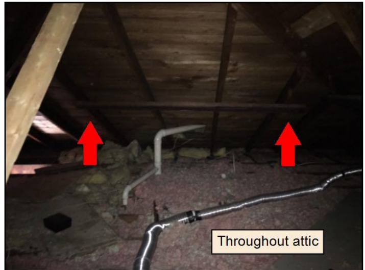
37. Purling Bracing Sagging/Damaged Location:...
