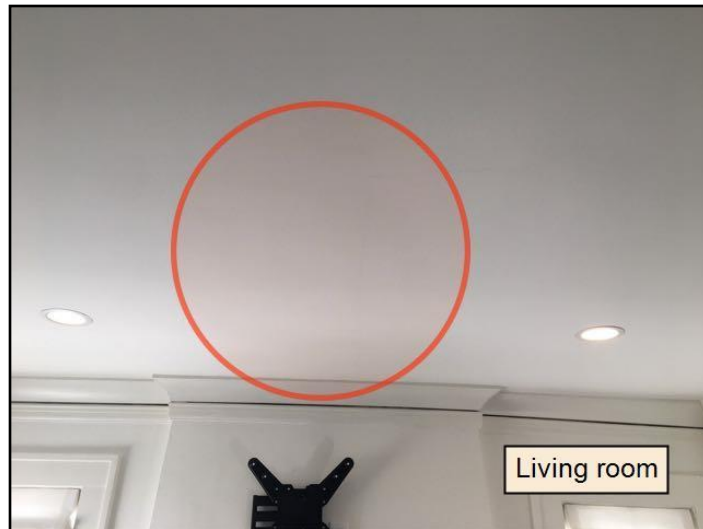
69. Water Stains Task: Request...
