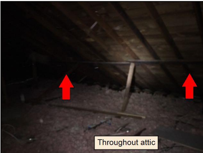
34. Purling Bracing Sagging/Damaged Location:...
