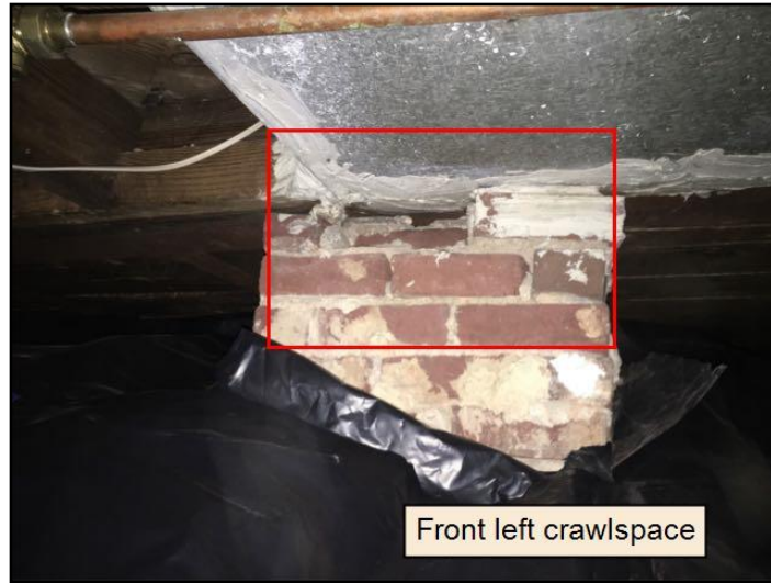
23. Mortar deterioration Task: Repair as...
