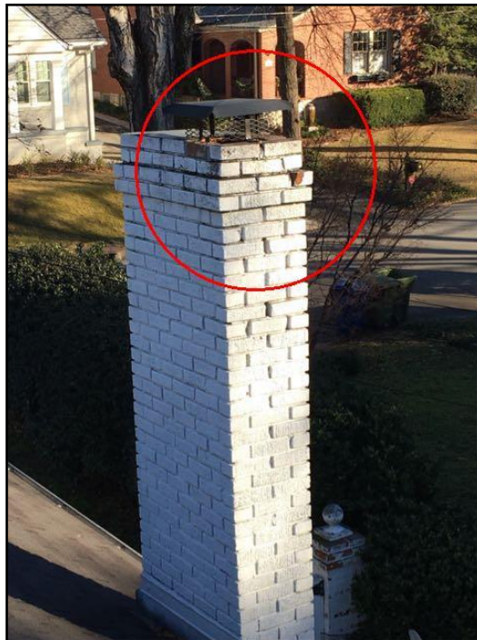
54. Loose, missing or deteriorated masonry
