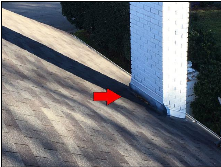
4. Cricket needed Location: Exterior roof at...
