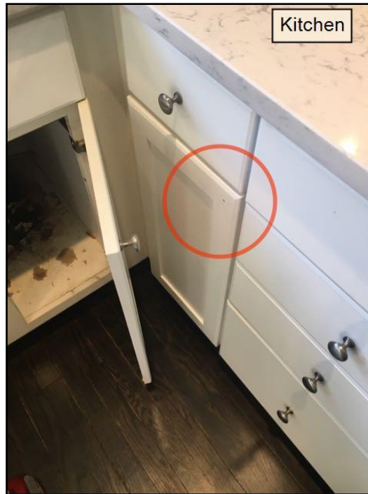
81. Pieces missing or loose
