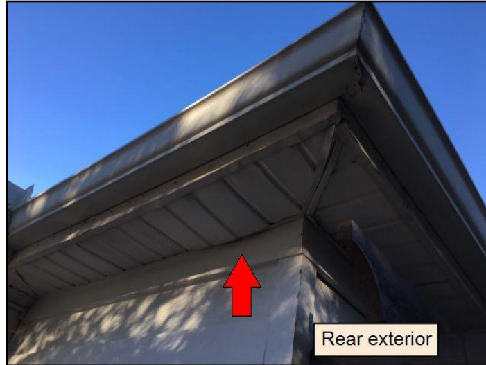
11. Loose/Missing pieces Task: Reinstall piece...
