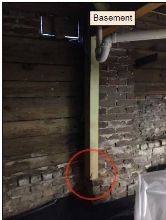
24. Poorly secured at top or bottom Task:...
