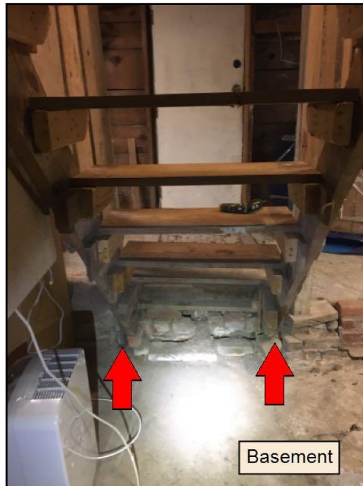
83. Poorly supported Task: Improve...
