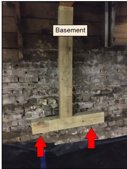
26. Poorly secured at top or bottom Task:...
