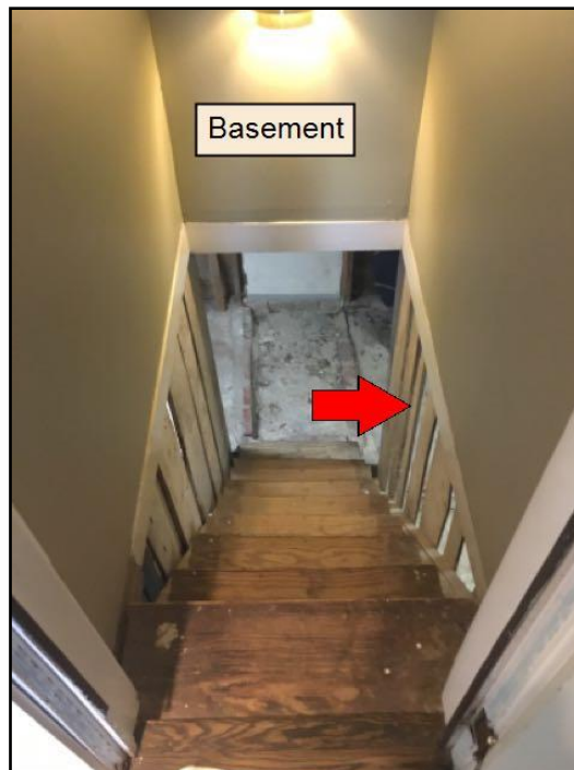
84. Missing Handrail Task: Provide Time:...
