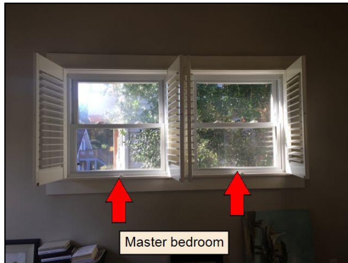
77. Sash Won't Stay Open Task: Repair Time:...
