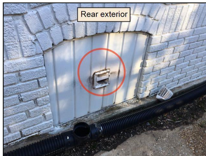
15. Vent cover damaged/missing Location:...
