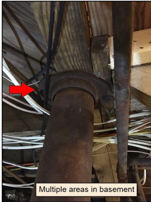
30. Poorly secured at top or bottom Task:...
