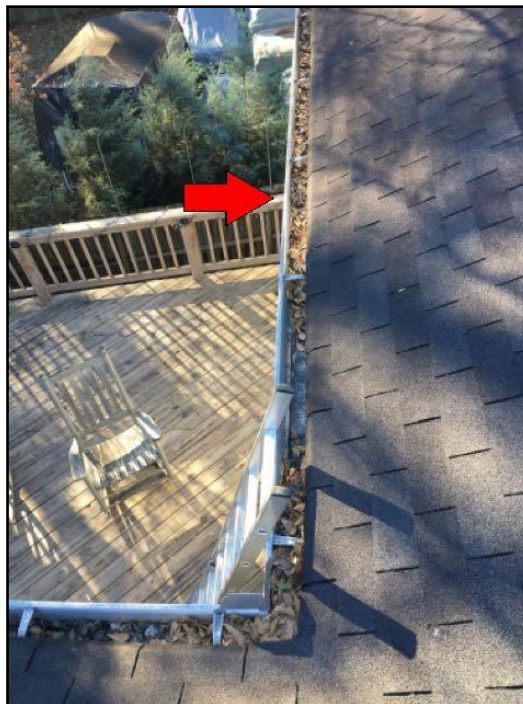
10. Clogged Location: Throughout...
