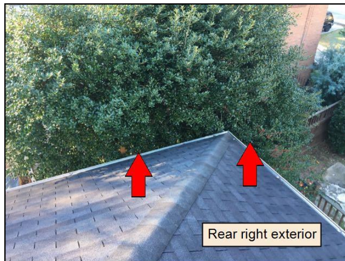
19. Trees or Shrubs too close to building Task...
