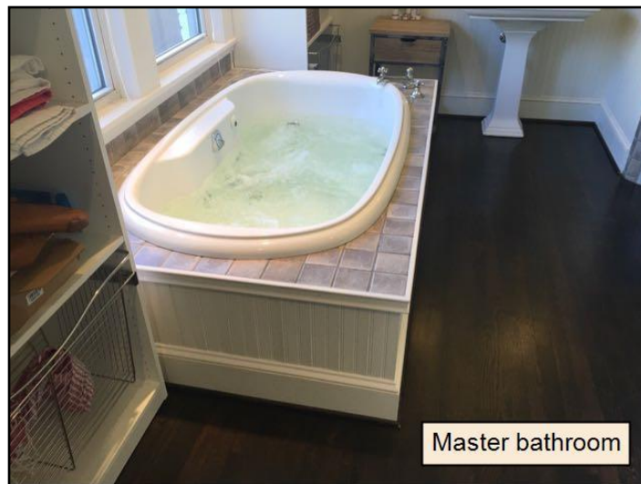
67. No pump access
