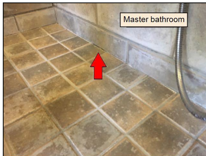
65. Caulking/Grout missing and or...
