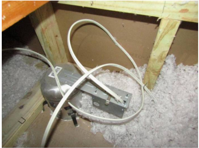
missing insulation above master bedroom
