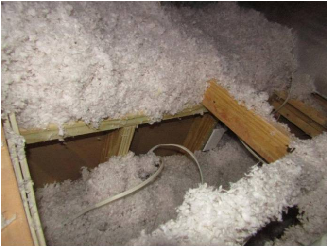
missing insulation above master bedroom
