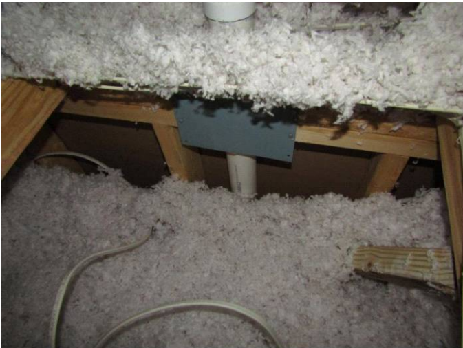
missing insulation above master bedroom
