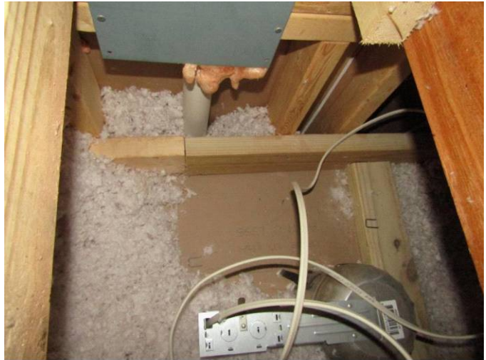
missing insulation above master bedroom
