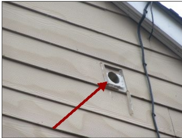
Damaged vent at the right wall
