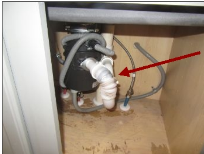
Improper flex drain below kitchen sink
