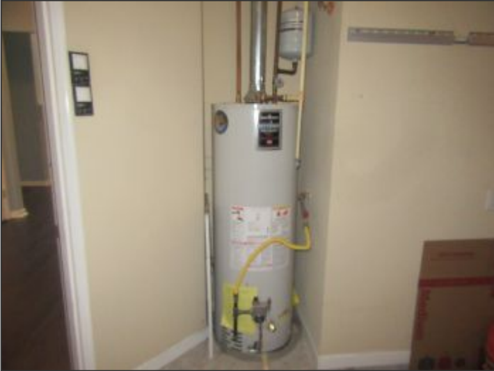
Water heater in the garage
