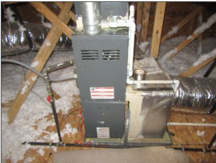
Second floor furnace in the attic
