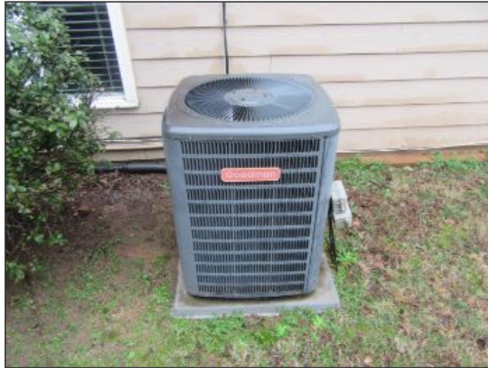
First floor AC unit
