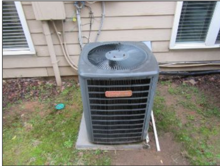
Second floor AC unit
