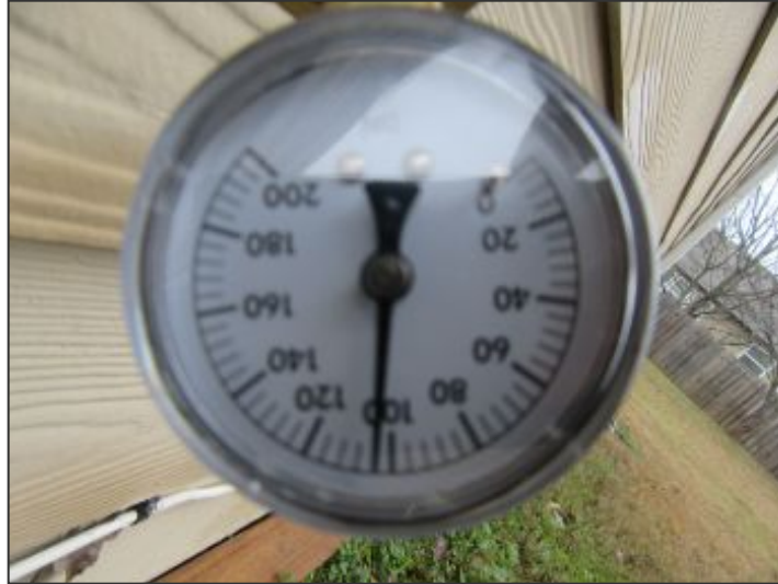
Water pressure is high at 105 psi
