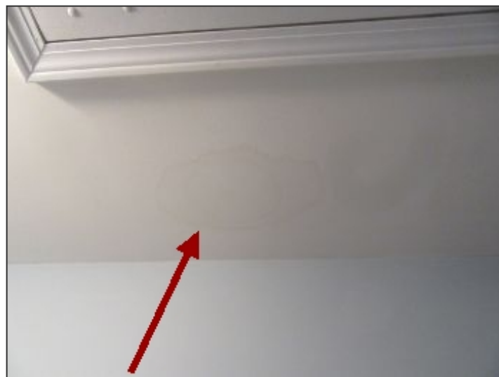
Water stain at the hallway near the attic ladder
