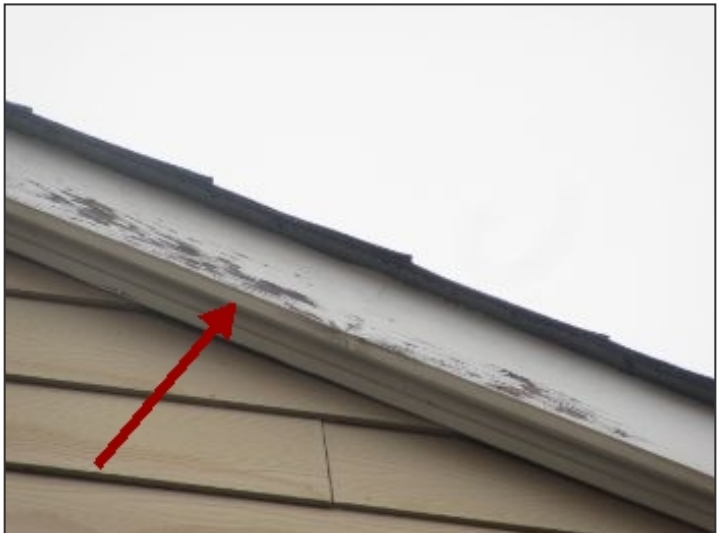
Peeling paint at the fascia boards
