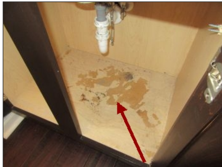
Damaged cabinet floor at the first floor bathroom
