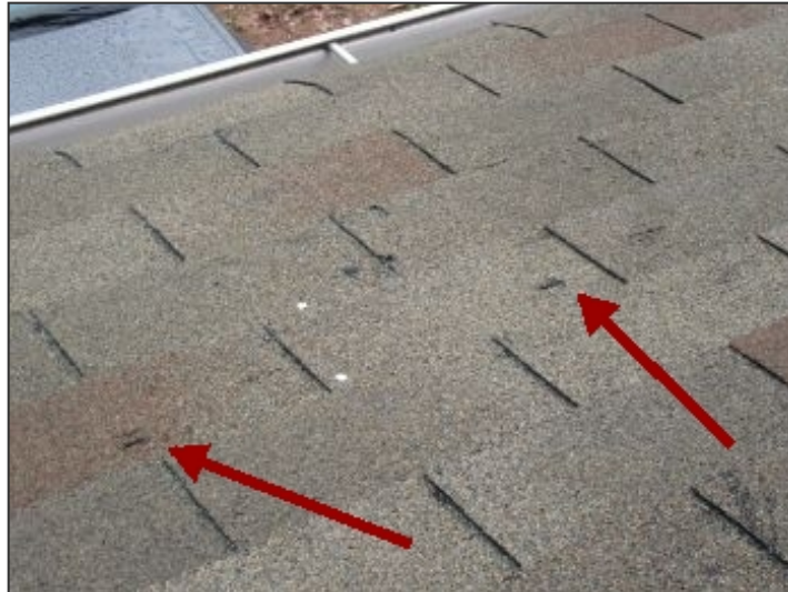
Shingle damaged at the front porch roof
