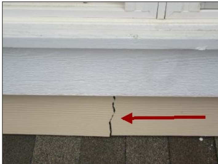
Damaged siding at the front wall above the front porch roof
