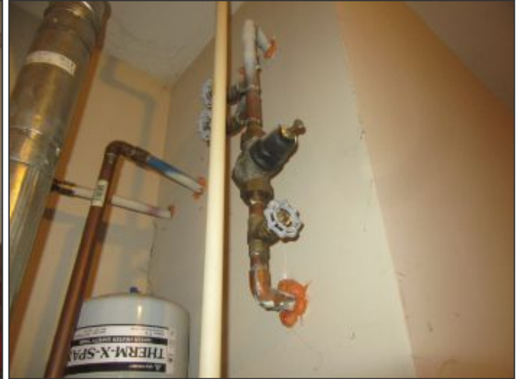
Main water cut off in the garage
