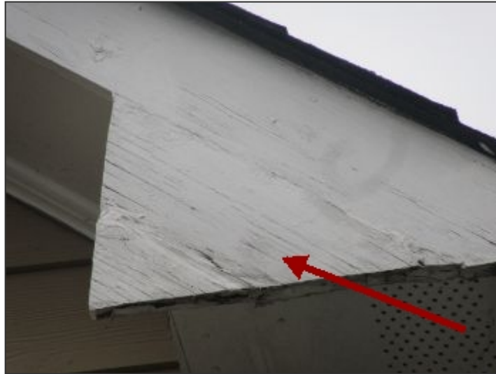
Damaged wooden fascia at the rear gable
