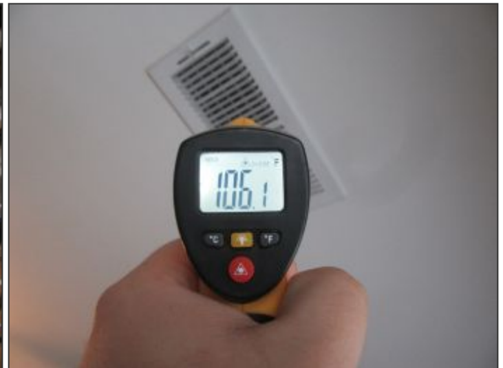
Second floor heating temps are normal
