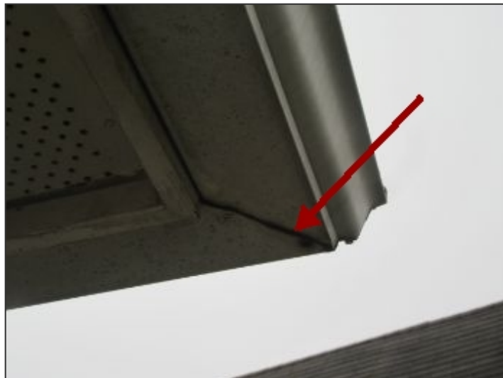
Gutter seam leak at the front gutters
