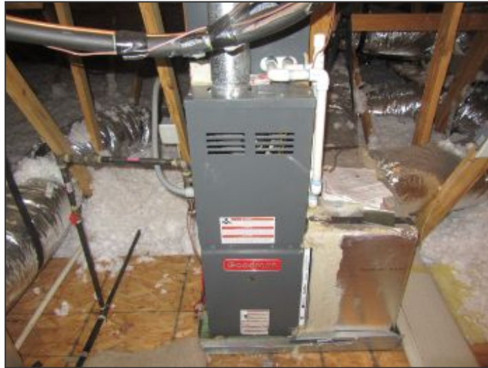
First floor furnace in the attic
