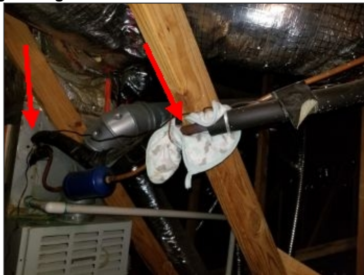
Coolant line not fully insulated in attic and at evaporator
