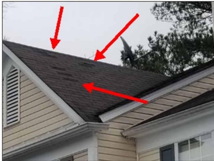
Missing shingles at front right gabled roof
