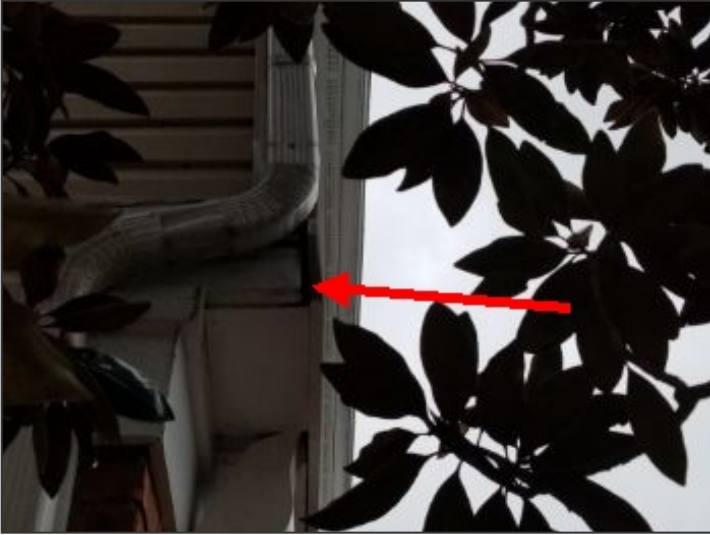
Open caulk joints at front left corner trim
