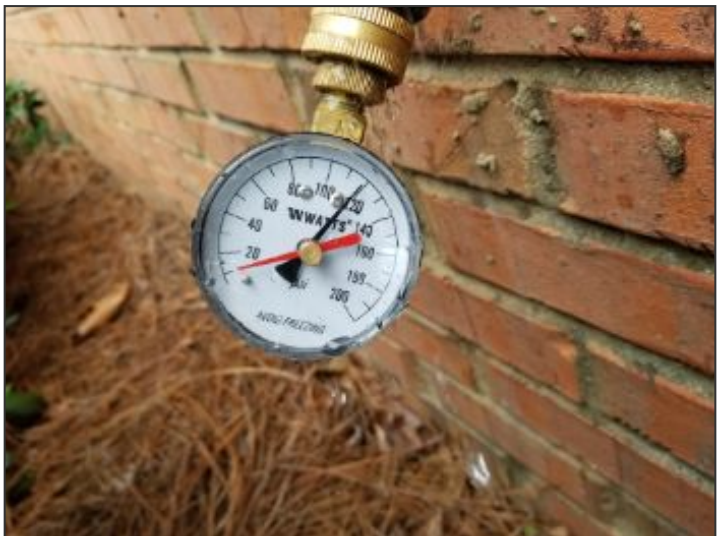
Water pressure too high at front hose bib
