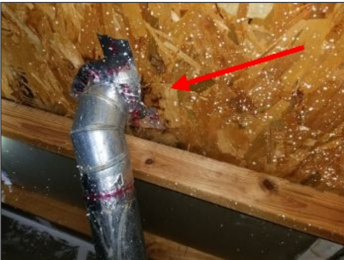
Evidence of a leak at laundry room dryer vent penetration
