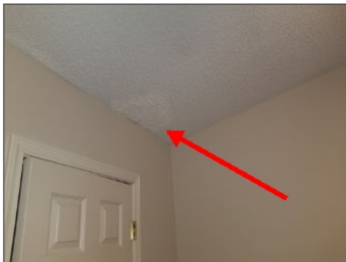
Ceiling / paint repair at master bedroom above bathroom entry
