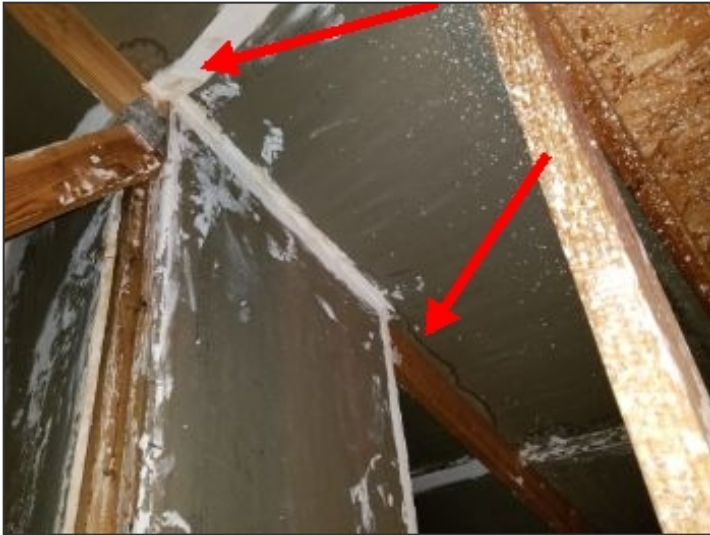
Evidence of a leak at chimney
