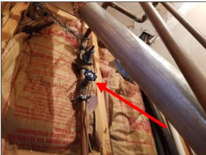
Main water cut-off handle located above water heater
