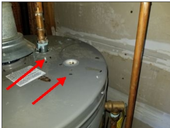
Rodent droppings on top of water heater in exterior closet
