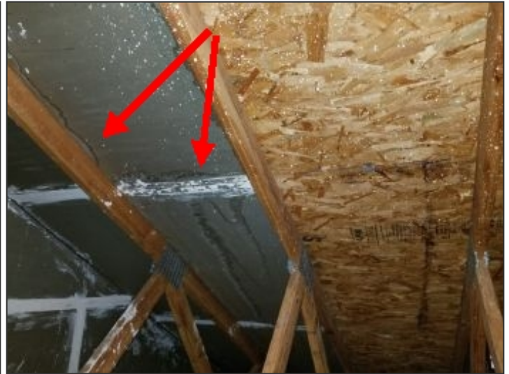
Evidence of a leak from chimney
