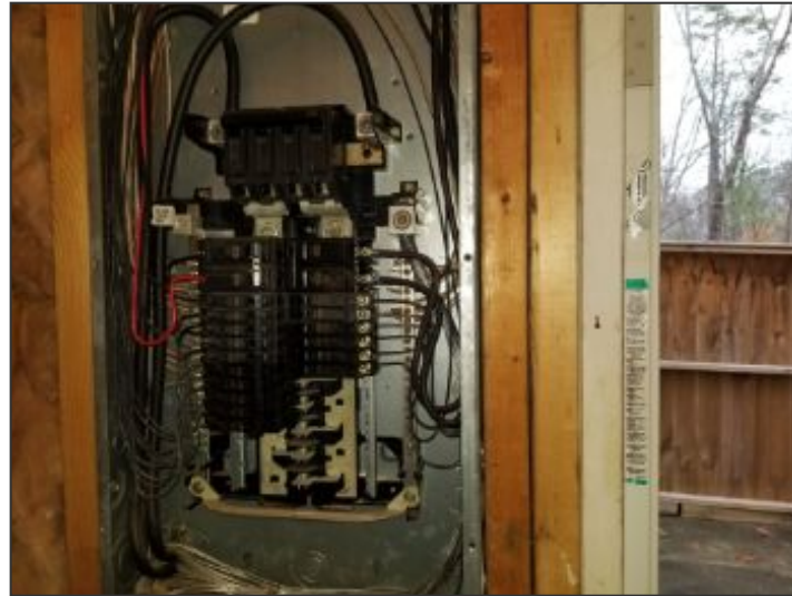
View inside main panel box
