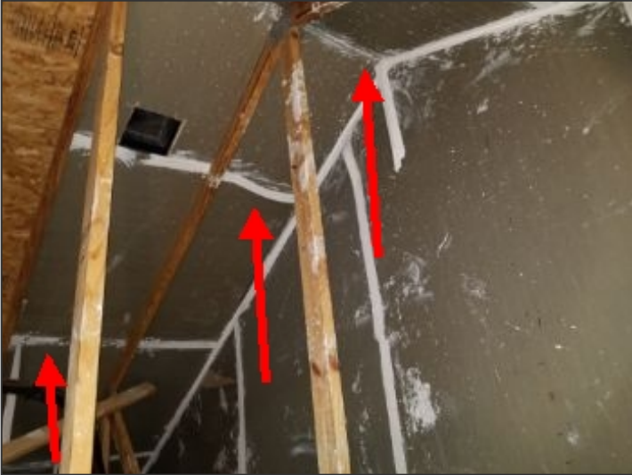
Loose sheetrock tape at fire walls
