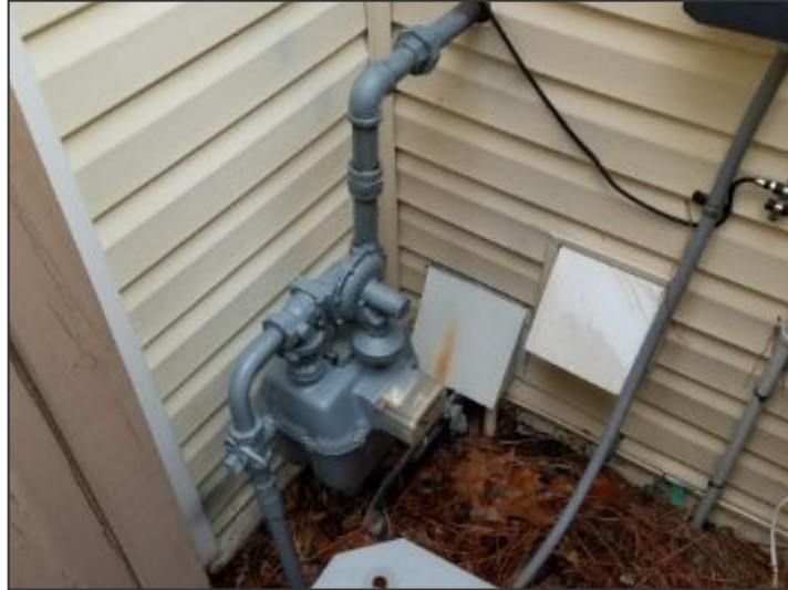
Gas meter at rear
