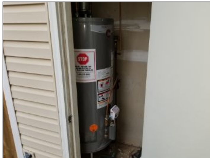
Water heater located in exterior closet
