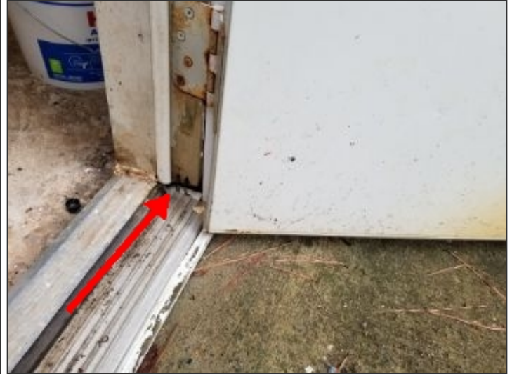
Moisture damaged wood at inside casing of exterior closet door
