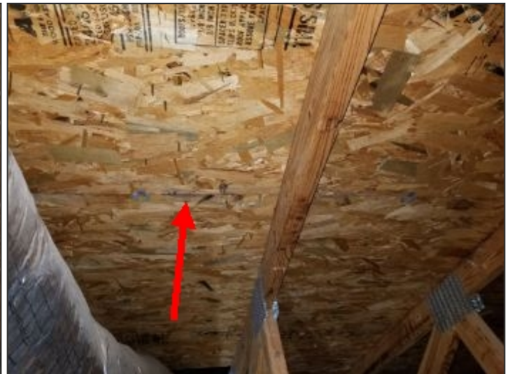
Evidence of a leak at front center roof above guest bedroom
