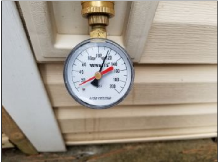
Water pressure too high at rear hose bib
