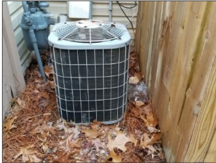
AC unit at rear
