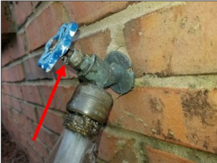
Active leak at turn handle when water is turned on at exterior hose bibs
