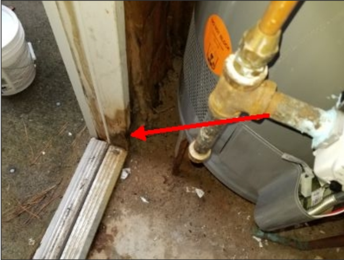
Evidence of water entry and damaged wood at rear exterior patio entry door
