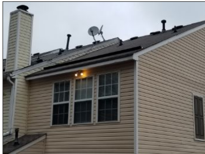
Recommend gutter installation at rear roof
