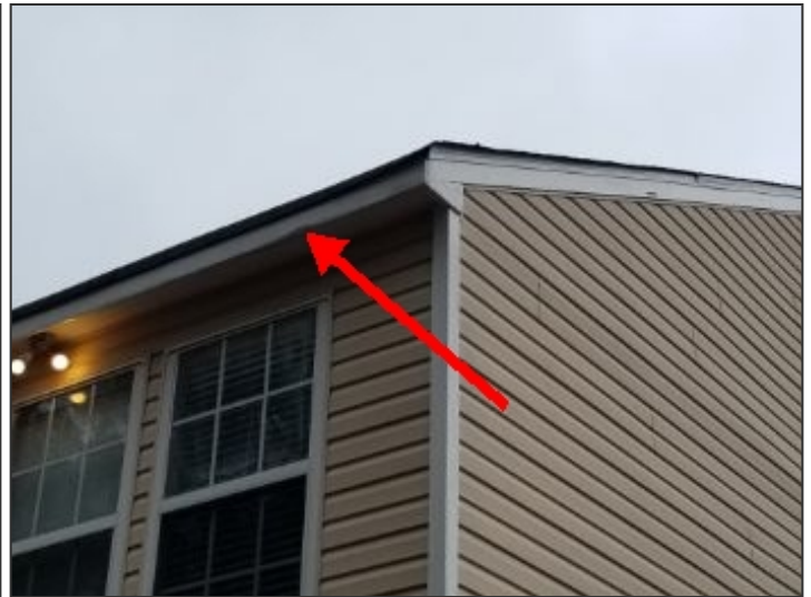
Damaged fascia at rear corner roof
