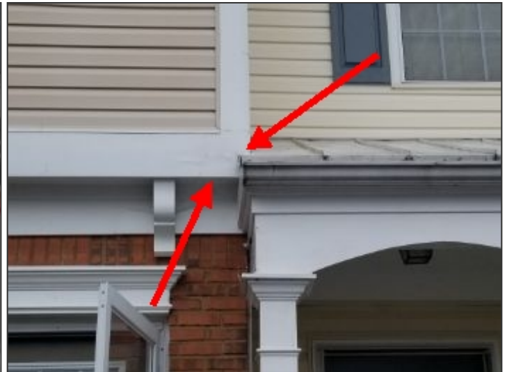
Damaged wood trim at front corner roof above adjoining metal roof
