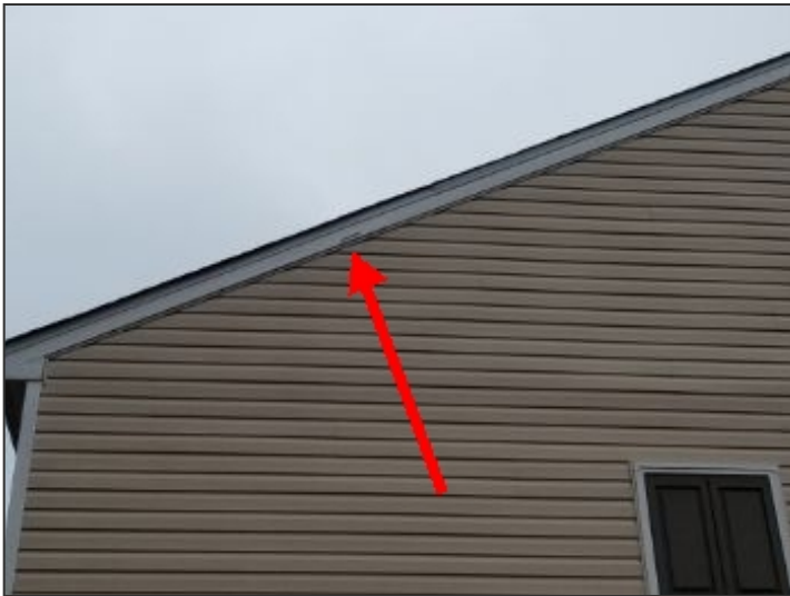
Damaged fascia at left side gabled roof
