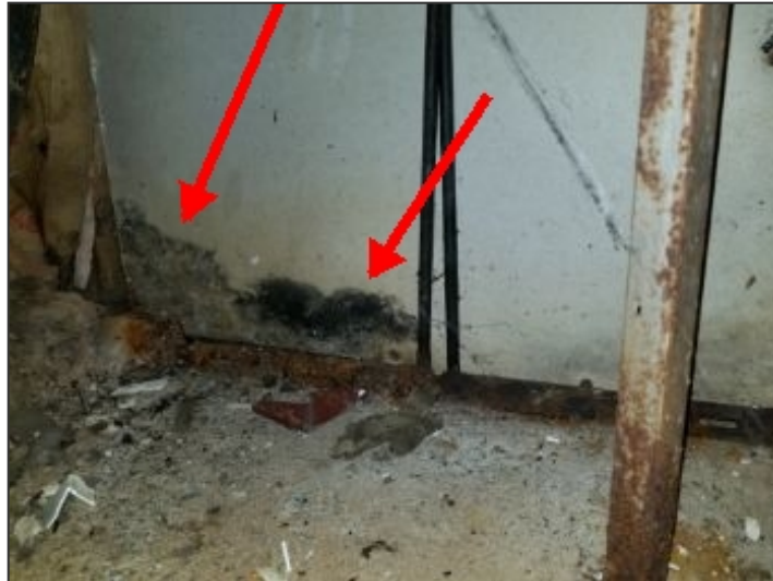
Suspected mold growth at lower sheetrock wall in exterior closet
