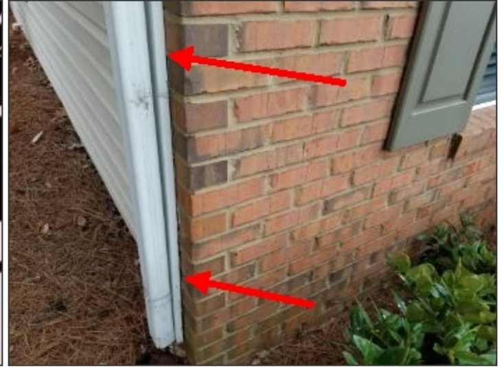
Caulk sealant missing at front left corner wood to brick location
