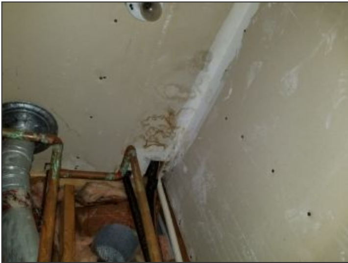
Water stains at exterior closet ceiling below coolant line
