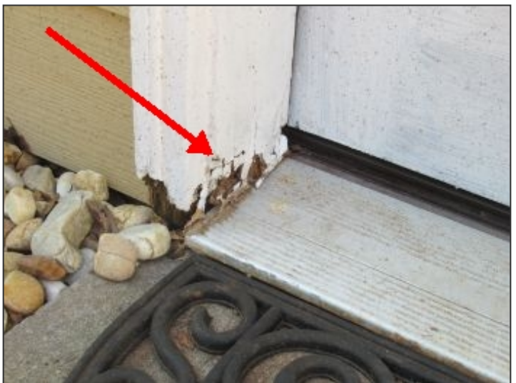
Water damaged trim at basement entry door
