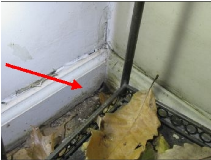
Signs of water entry at front garage wall, damaged baseboard
