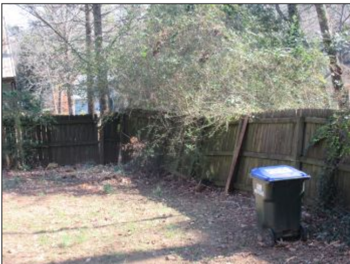
Leaning fencing at rear corner yard
