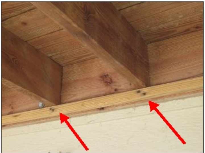
Joist hangers are recommended at porch
