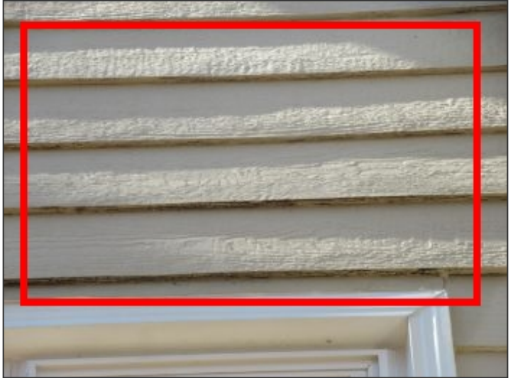
Damaged siding at rear wall
