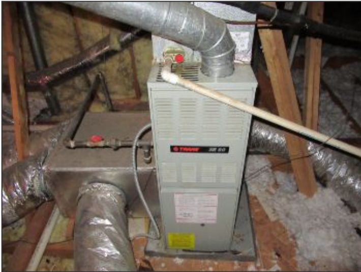
Second floor furnace in attic - 1994
