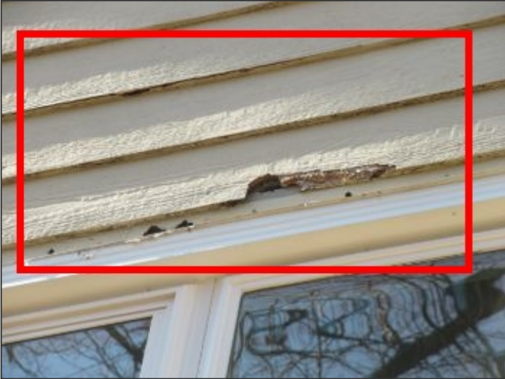
Damaged siding at rear family room
