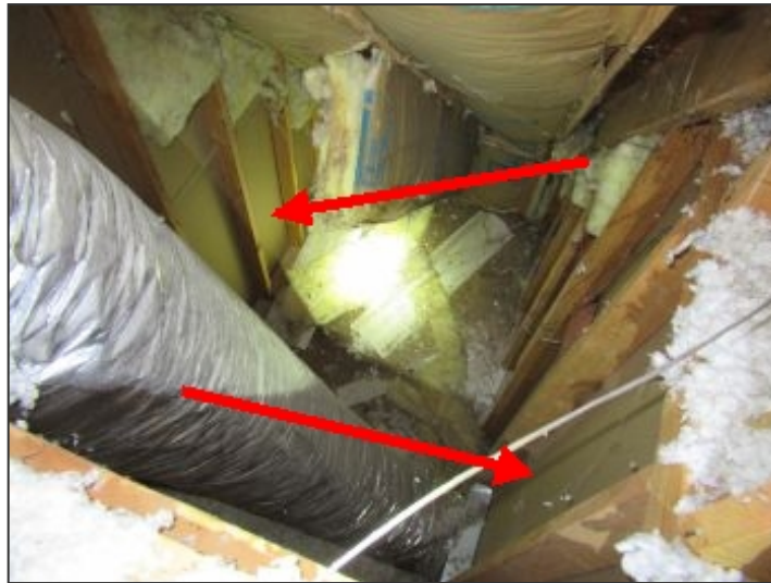
Missing wall insulation at front attic near master
