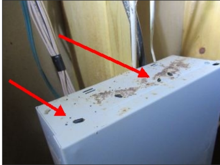
Rodent droppings on box below stairs
