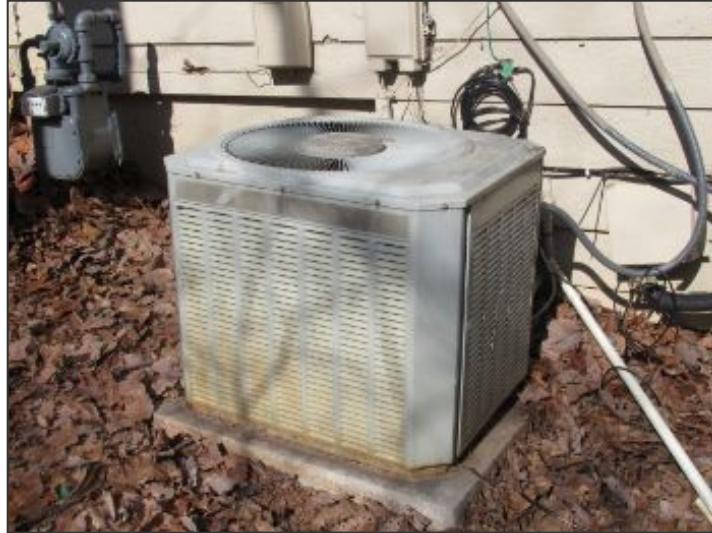
Second floor AC unit - 1994
