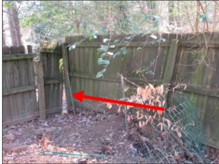
Openings at rear corner fencing
