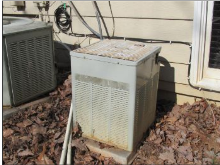
First floor AC unit - 1994
