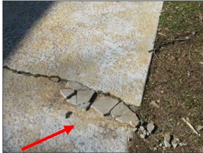
Damaged concrete at driveway parking pad
