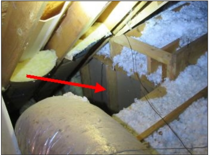
Missing attic insulation on master bedroom wall near thermostat
