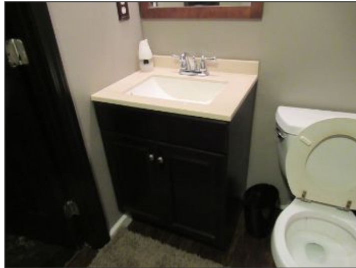
Basement bath vanity cabinet is loose, unsecured
