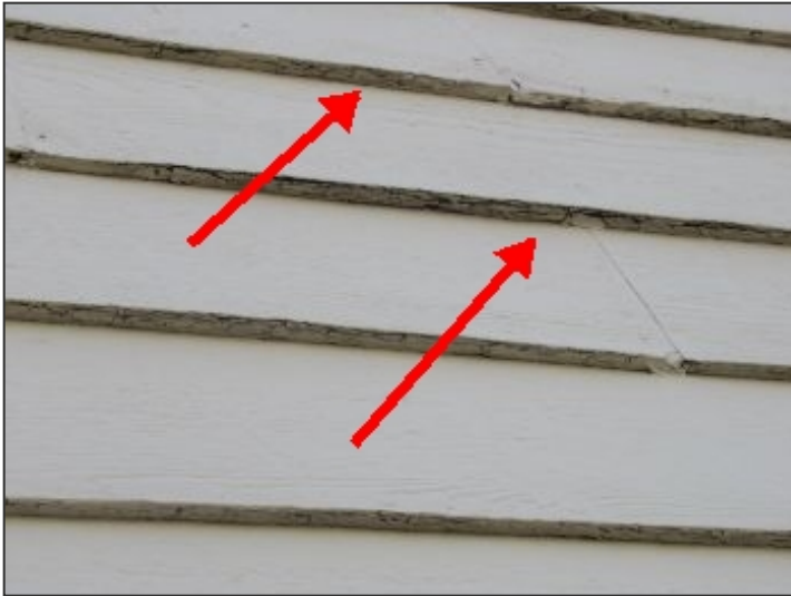
Moisture damaged siding boards above garage doorway
