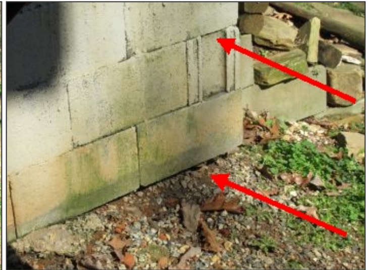
Retaining wall has no mortar and no footings
