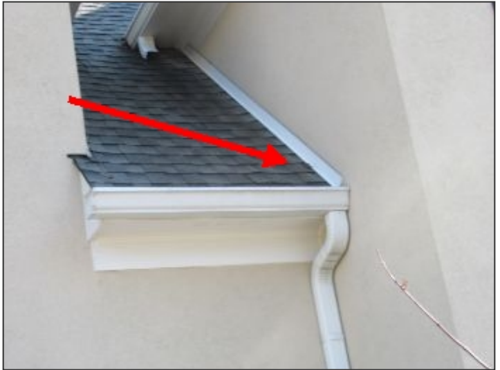
No kickout flashing at stucco wall and roof
