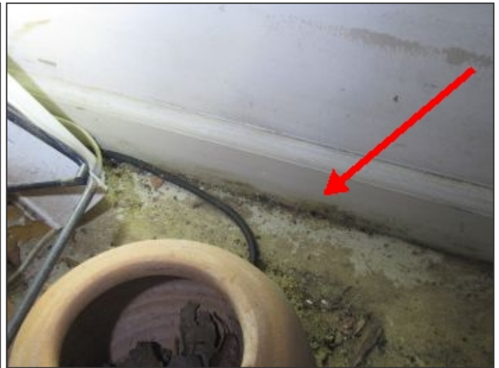
Water staining at front garage wall
