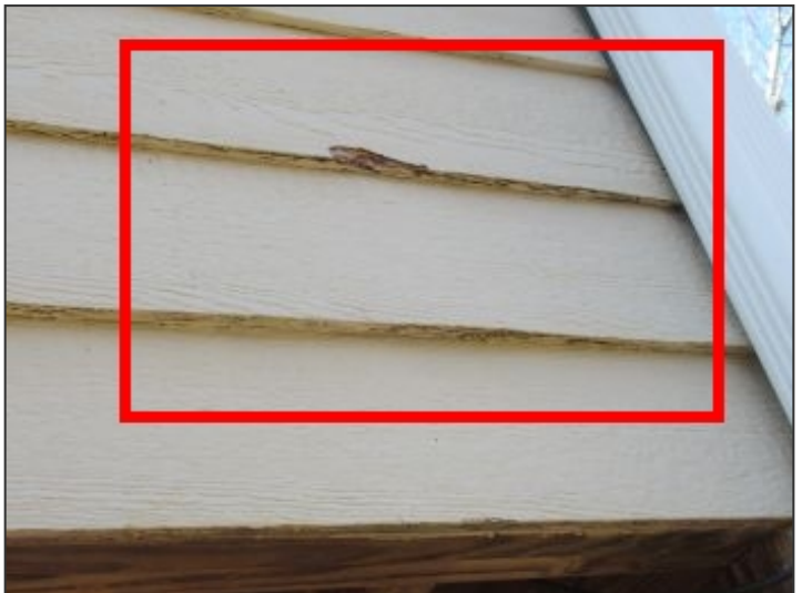
Damaged siding at rear porch wall
