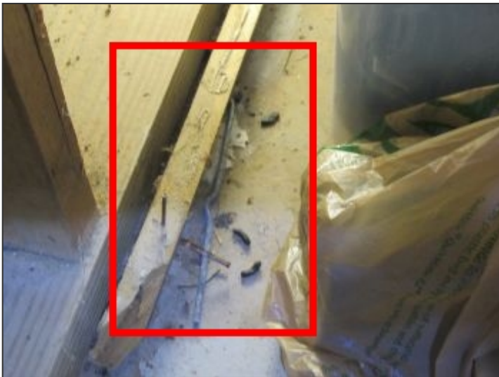
Rodent dropping on floor below stairs
