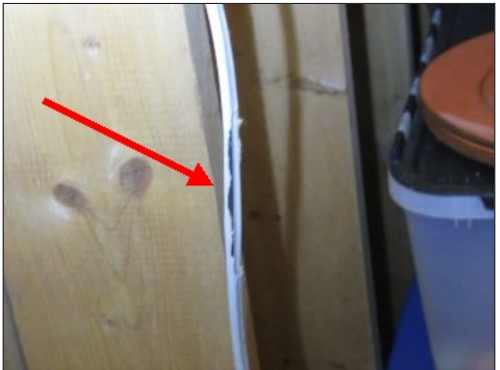
Rodent chewed electrical wiring below basement stairs
