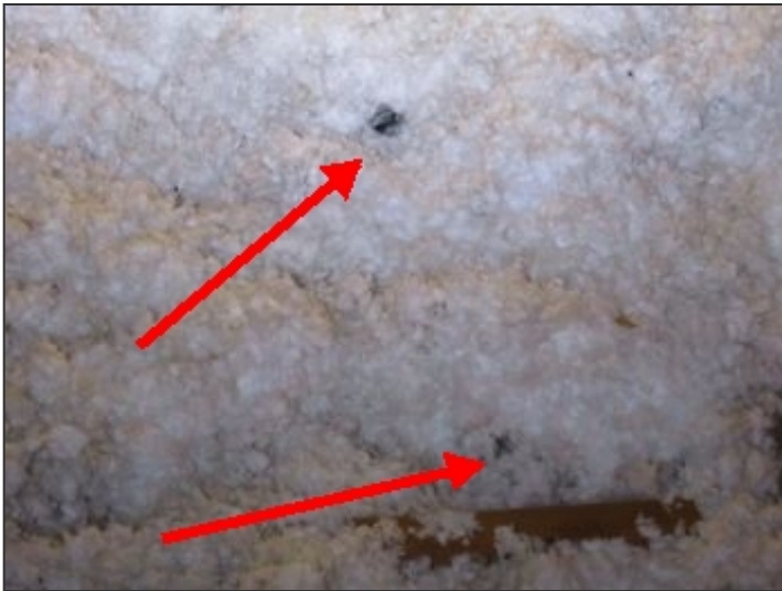
Rodent tunnels in attic insulation
