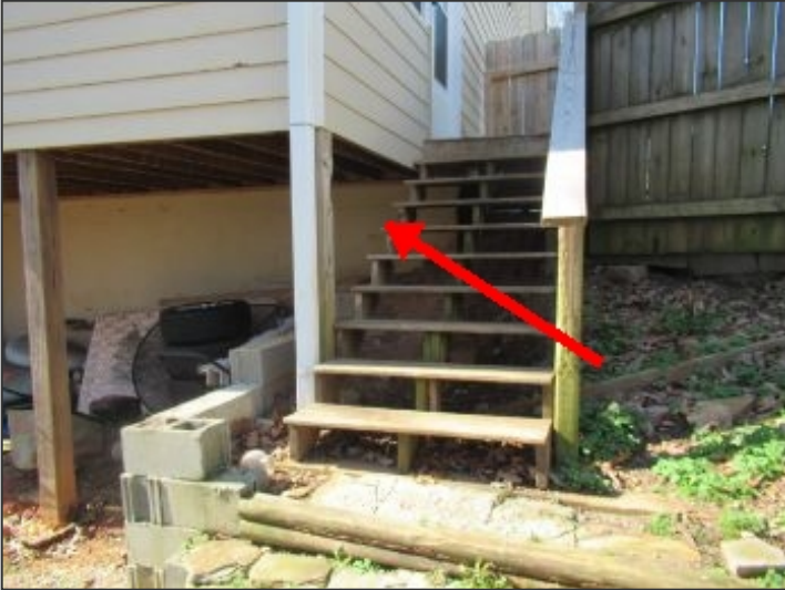
Unsafe condition at rear stairs - missing railings
