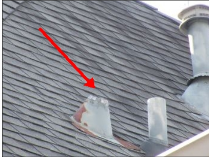
Laundry dryer vent is missing vent cap, has been sealed off
