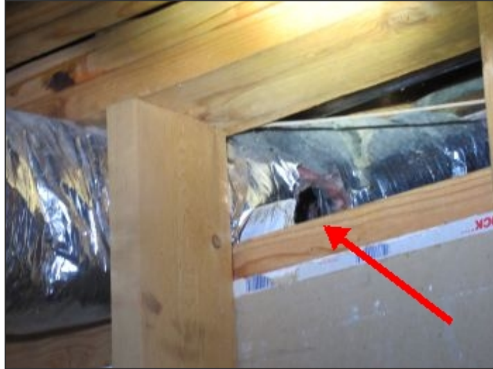
Large hole in HVAC duct in basement mechanical room ceiling
