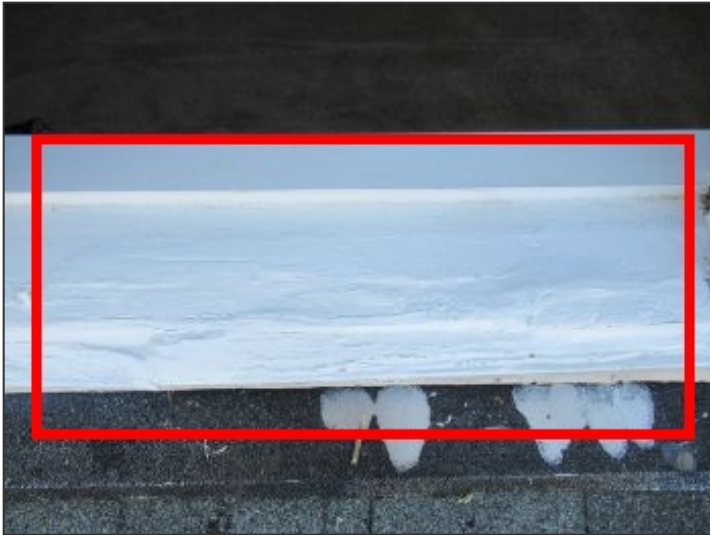
Severe water damage at rot at rear master windows
