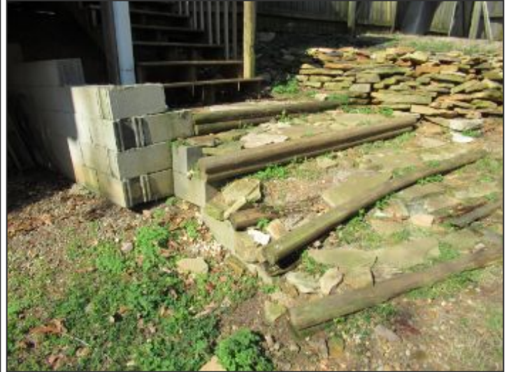
Unsafe condition: damaged and loose timbers at bottom of stairs
