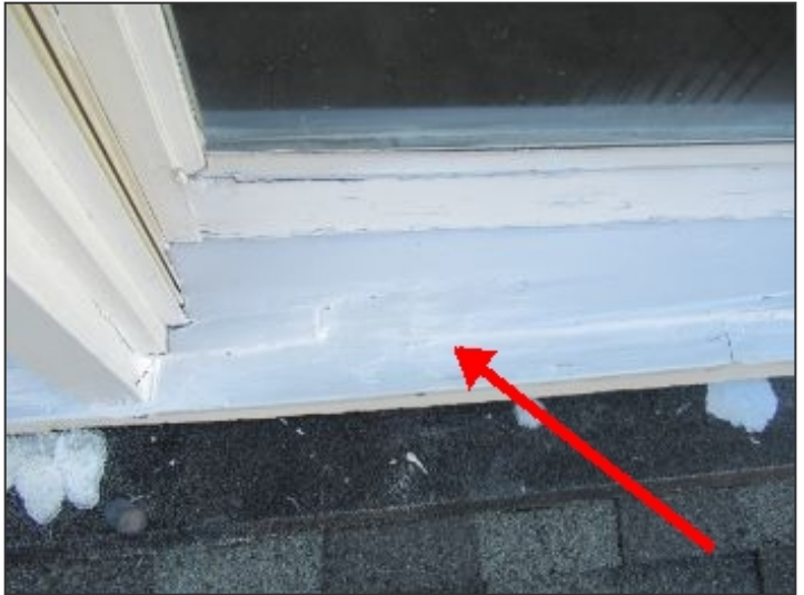
Severe water damage at rot at rear master windows, inadequate patch repairs
