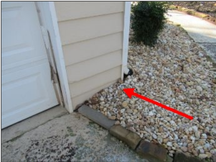
Soil and stones are too high above siding and trim
