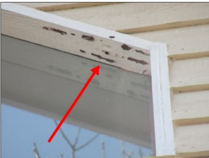
Insect damage at rear master bath windows
