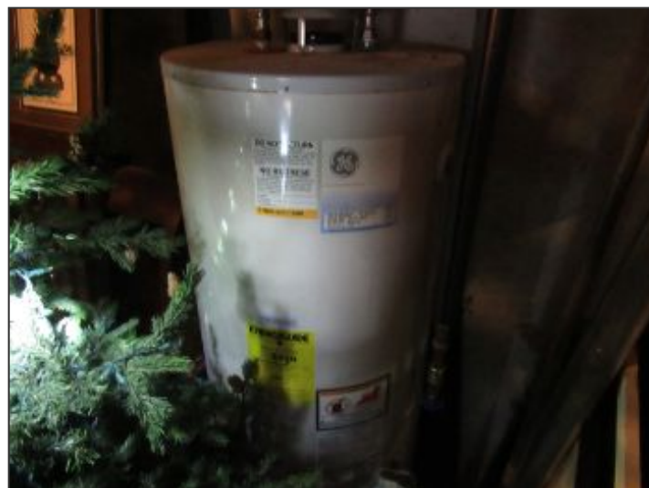
Water heater in basement - 2010
