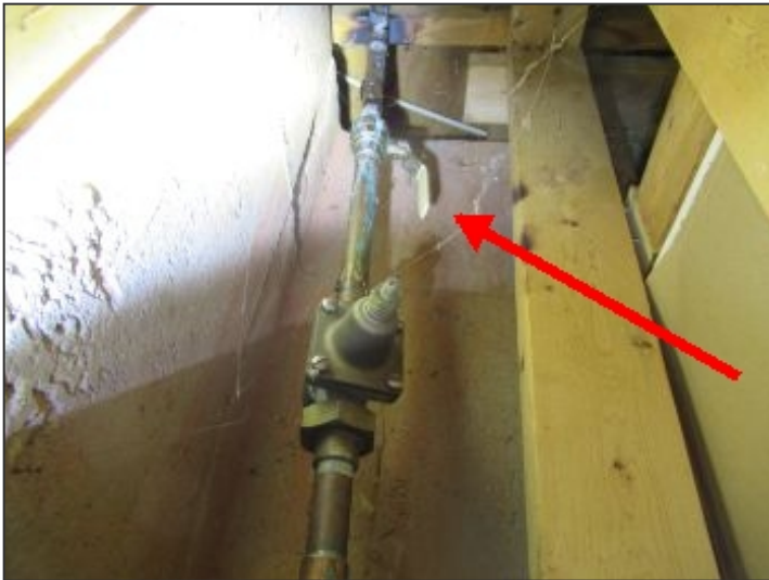
Main water cutoff at front basement
