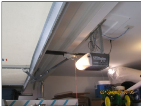
Liftmaster 1/3HP chain drive opener noted.
