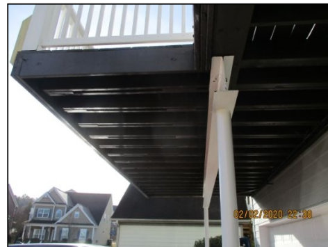
Settlement noted on outer rim band of deck because steel I-Beam is not located in middle to outer section.
