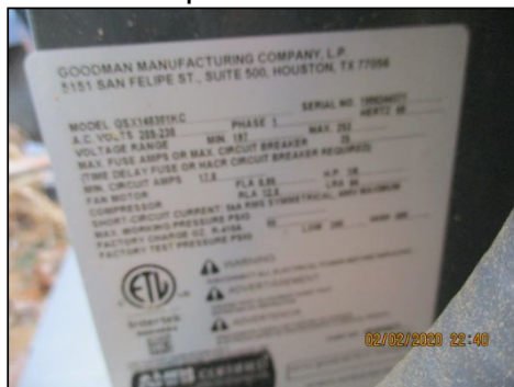
Goodman 2013, 2.5 Ton AC compressor noted.
