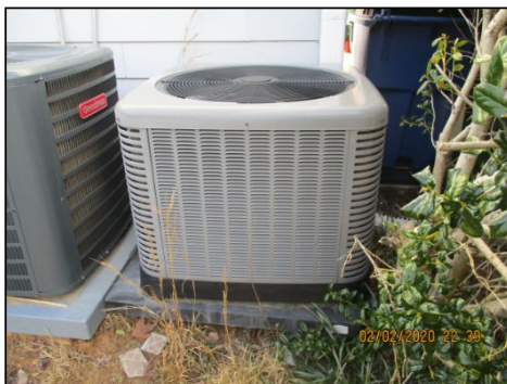
Rheem 2015, 3 Ton AC compressor noted.
