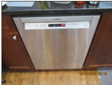
Bosch dishwasher noted. Operated properly when tested.
