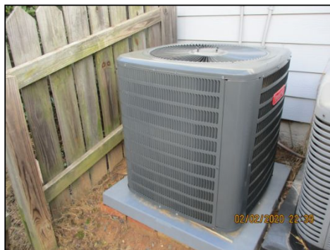
Goodman 2013, 2.5 Ton AC compressor noted.
