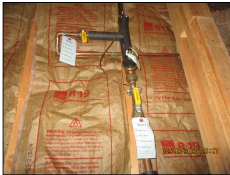
Pressure regulator noted in main water line in basement.
