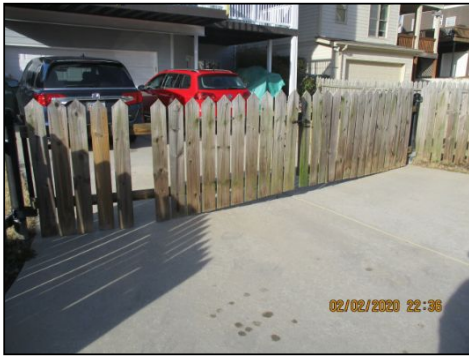
Driveway gate is in good condition with missing slats noted.
