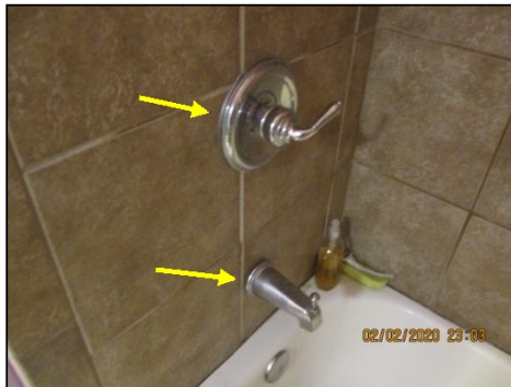
Recommend securing loose plumbing valve and faucet in basement shower to prevent leaks.
