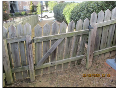
Broken gate noted on right side of house. Recommend licensed contractor to evaluate and repair gate as necessary.
