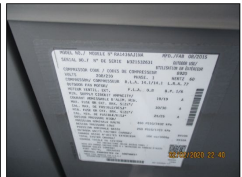
Rheem 2015, 3 Ton AC compressor noted.
