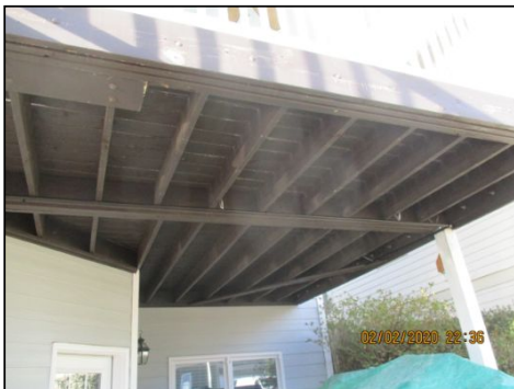
When deck was built code did not permit for joist hangers to be used as supports. Recommend decking company to install joist hangers instead of 1x2 rail that is supporting deck joists.
