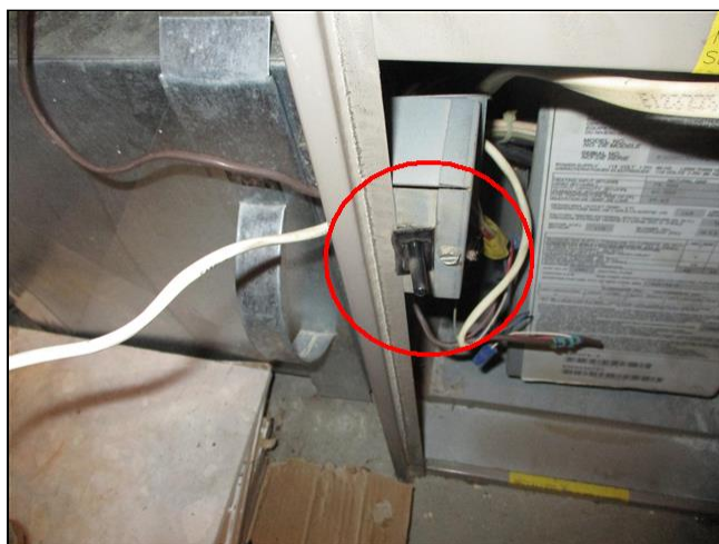
6.0 Item 4(Picture) blower door switch
