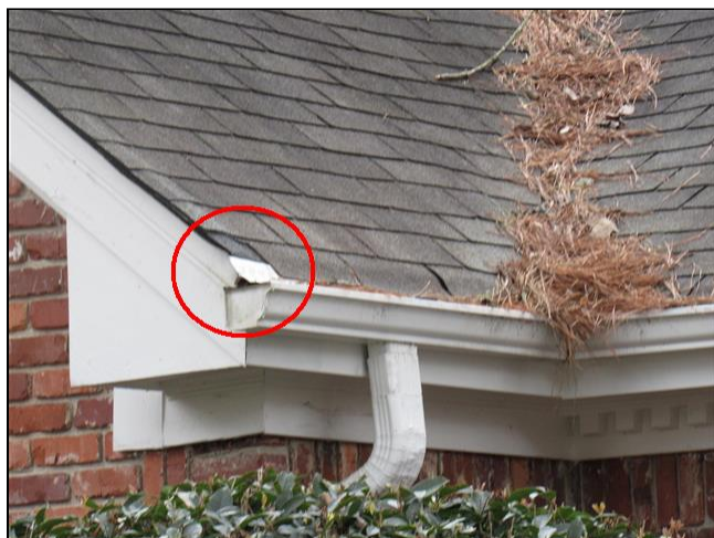
4.0 Item 7(Picture) missing shingle
