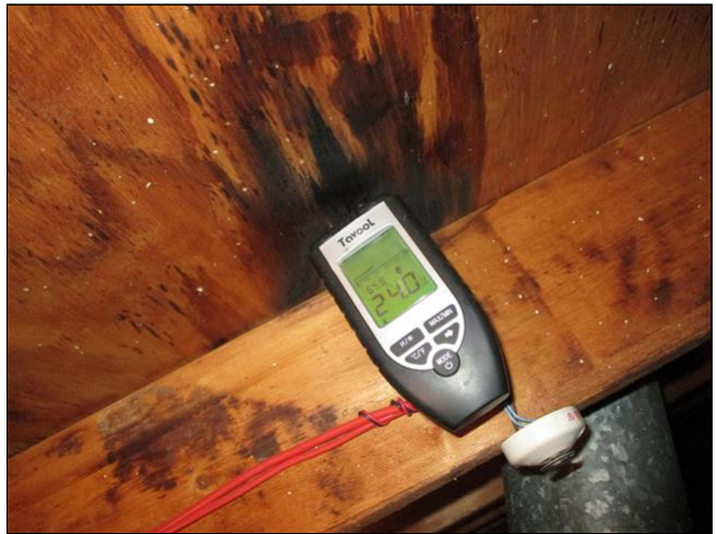
4.4 Item 8(Picture) high levels of moisture near the gas exhaust vent
