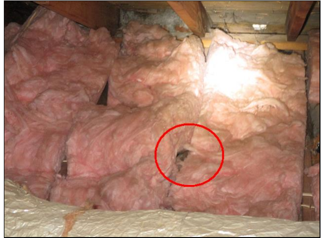
9.8 Item 2(Picture) rodent tunnel
