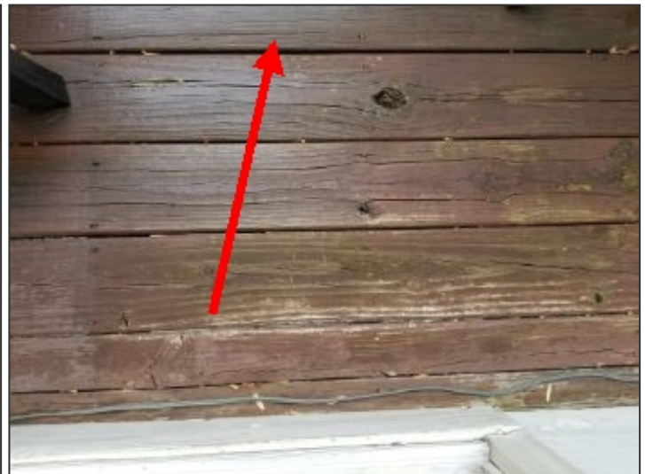
Damaged deck surface board
