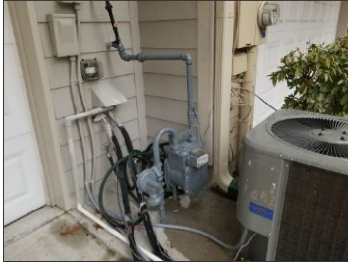
Gas meter at rear wall
