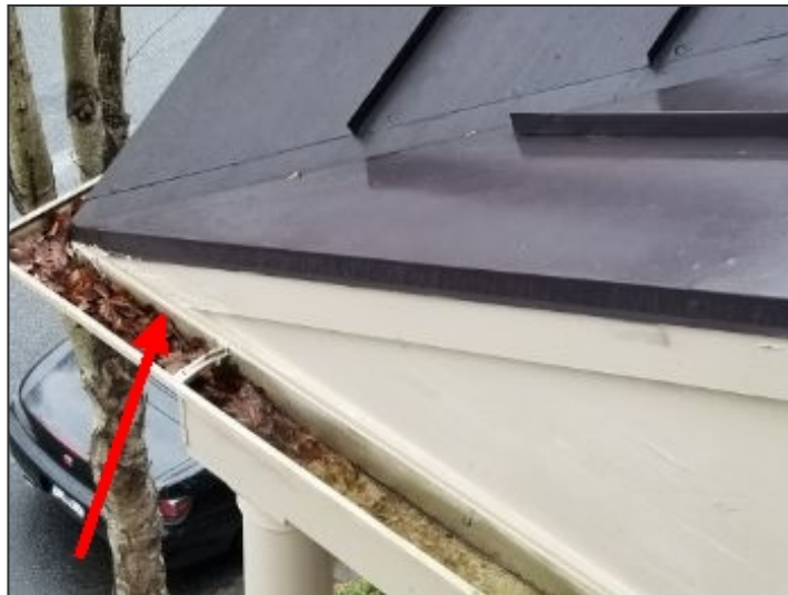
Damaged wood trim at right corner of porch roof
