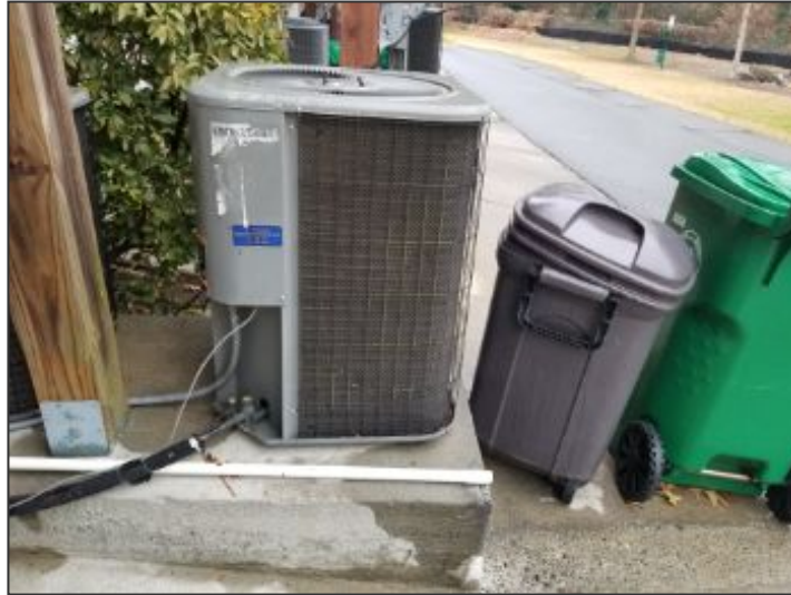
Main floor and lower level AC unit
