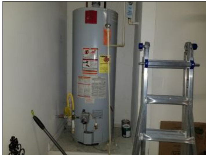
Water heater located in garage
