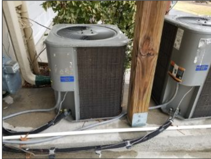
Second floor AC unit
