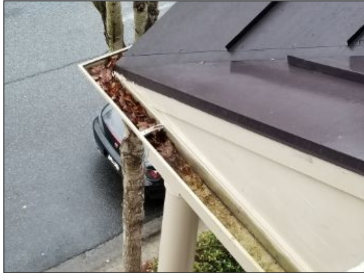
Gutter debris at front porch roof
