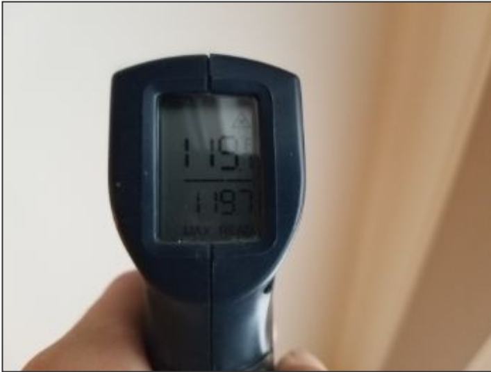
Good temps during testing of main floor furnace
