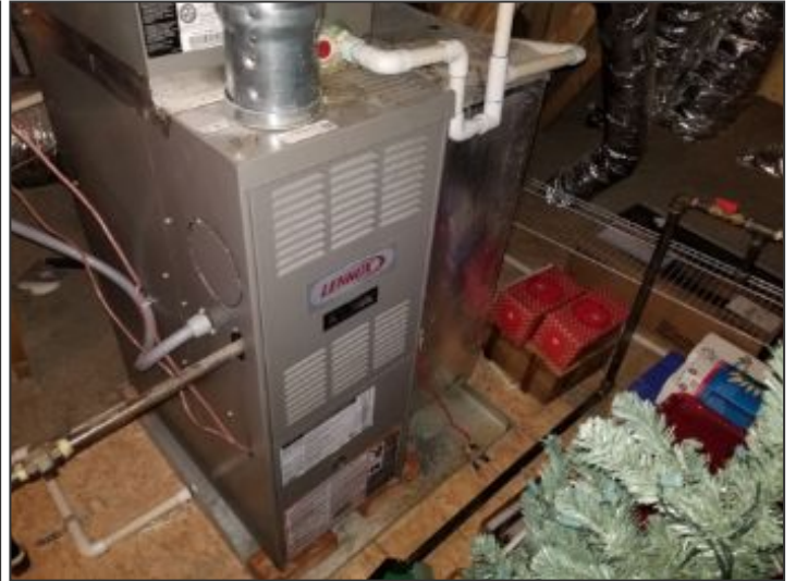
Second floor furnace located in attic
