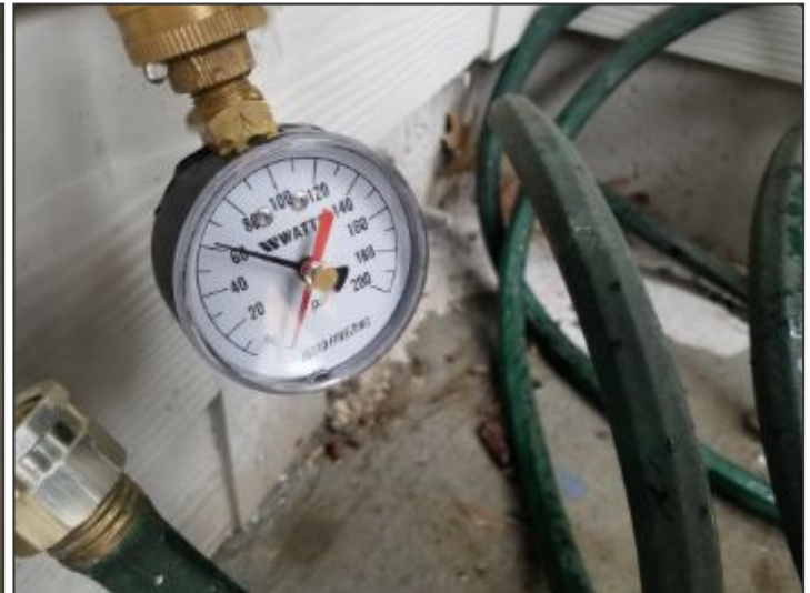
Water pressure normal at 62 PSI
