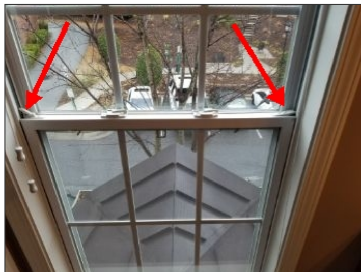
Damaged tilt-out lock at front upstairs bathroom window
