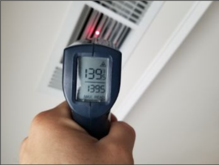
Good temps during testing of second floor furnace
