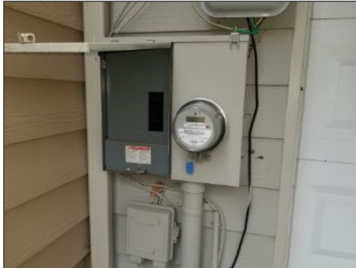
Main electrical disconnect at exterior meter
