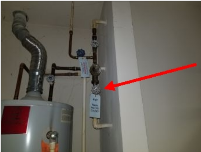
Main water cut-off handle located in garage
