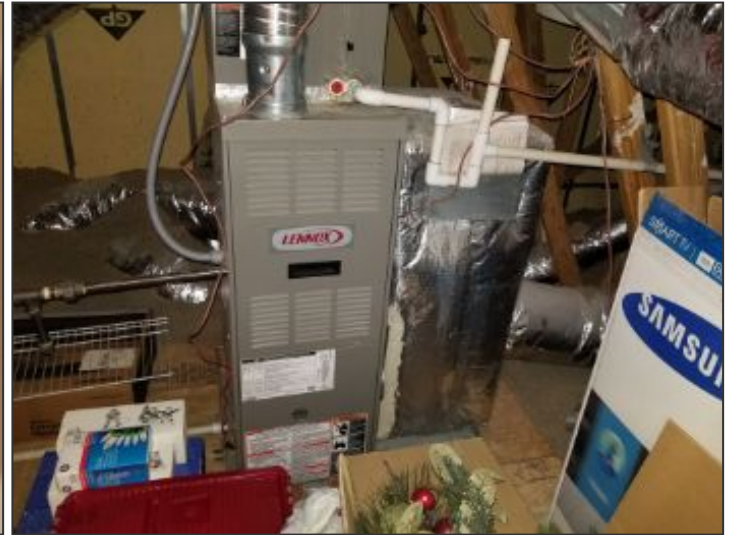
Main floor furnace located in attic Second
