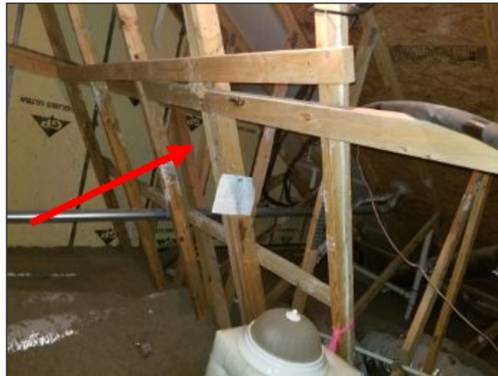
Damaged roof truss in attic partially braced
