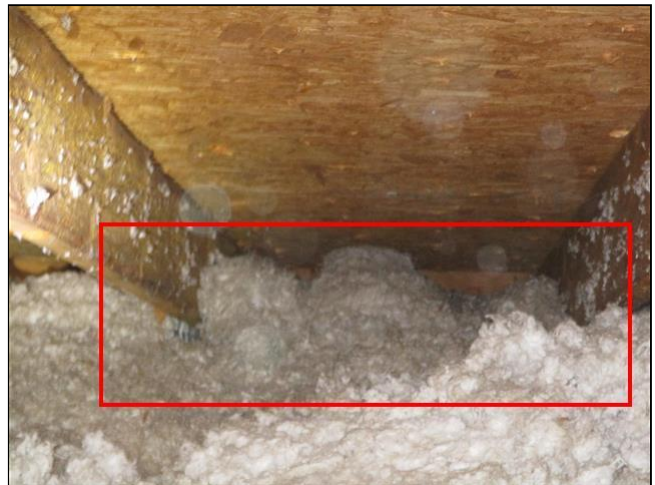
9.8 Item 2(Picture) rodent trails in attic insulation
