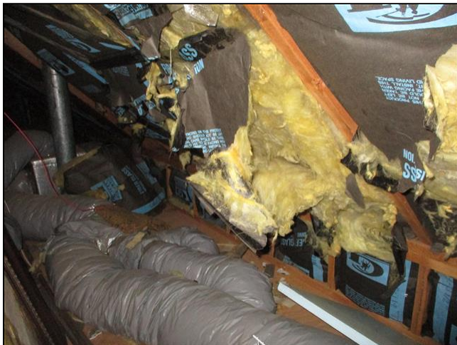
9.8 Item 1(Picture) chewed batts insulation
