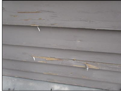
Paint weathered and peeling on the siding
