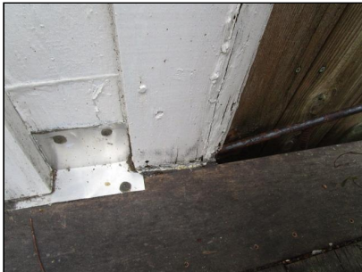
Repair all damaged trim
