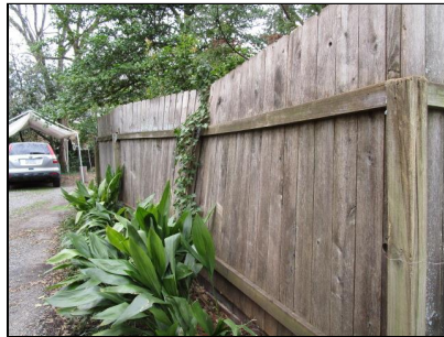
Secure the loose fence post at the rear of the house.
