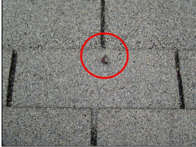
Nail pops penetrating shingles.
