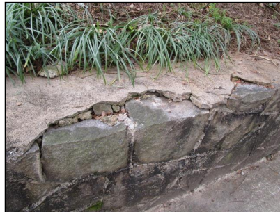
Extensive deterioration of the exterior front retaining wall.
