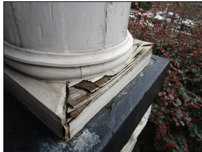
Repair all damaged trim
