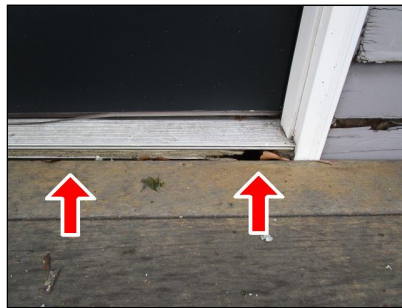
Deterioration of the rear door sill.
