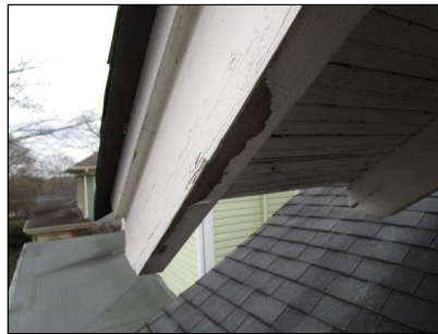
Paint weathered and peeling
