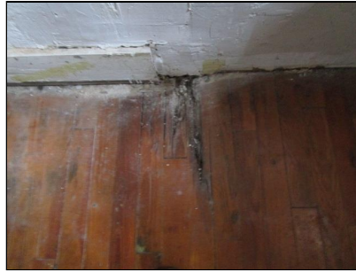
Damaged flooring in the rear closet.
