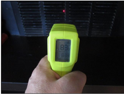
Emergency heat tested and functional.
