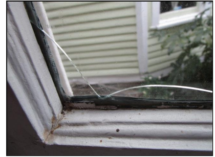
Replace all cracked window panes.
