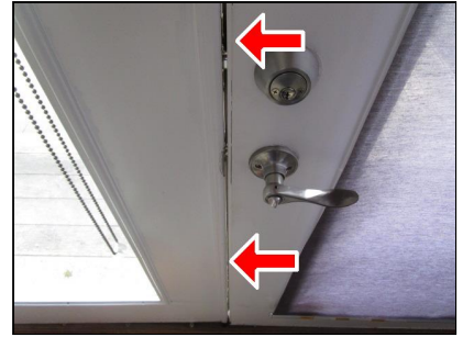
Daylight visible between doors.
