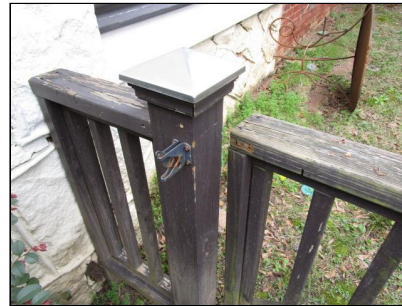
Repair all gates to latch properly.
