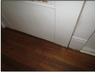
Front door sticks at the sill.
