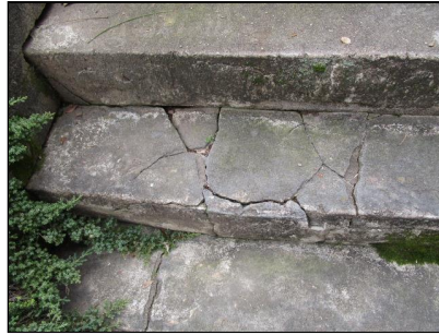
Repair cracked front stairs.
