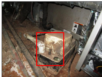
Drain line not properly connected to the pump.
