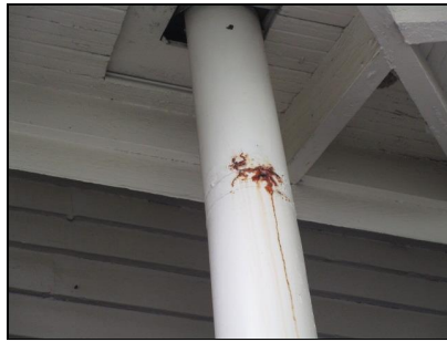
Flue rusting through on the exterior of the house.
