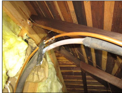
Add insulation in the attic where missing
