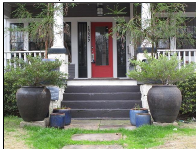
Add handrail to the front porch steps.
