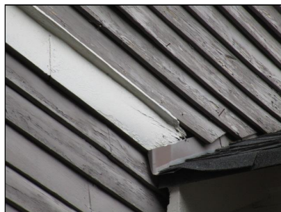
Repair all damaged trim
