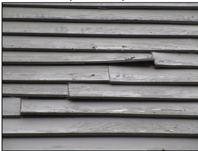
Replace all warped and damaged siding
