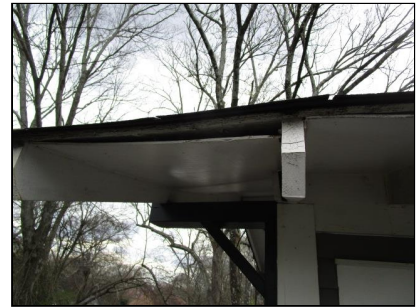
Damaged decking around perimeter of the roof.
