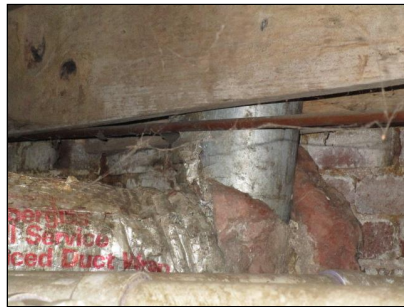
Add insulation to all ducts where damaged or missing
