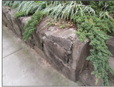
Retaining wall leaning and cracking.
