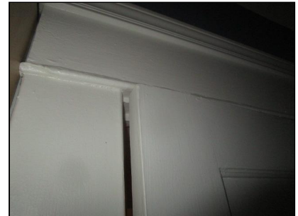
Doors stick in the frame, do not close and latch properly
