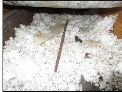
Signs of rodents in the insulation.
