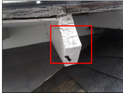
Repair all damaged trim
