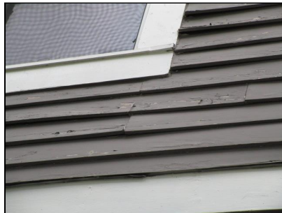
Paint weathered and peeling on the siding
