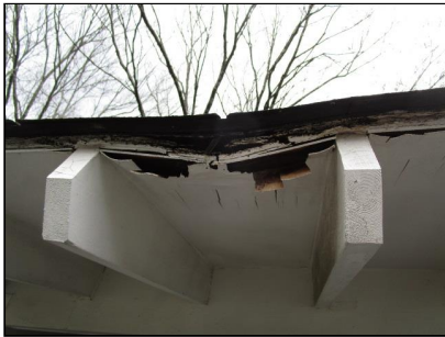
Damaged decking around perimeter of the roof.
