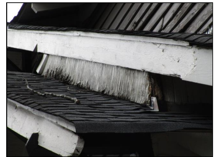
Replace all damaged siding
