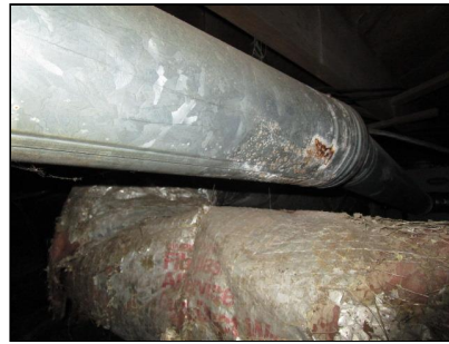
Flue rusting through in the crawlspace.
