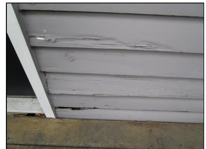
Replace damaged siding
