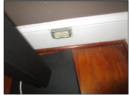
Replace missing cover.
