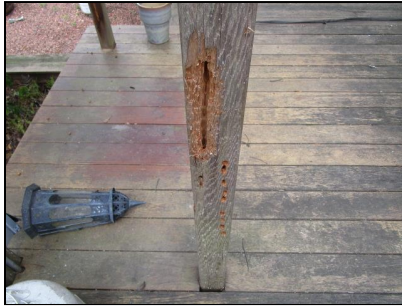
Repair carpenter bee damage to the deck roof support posts.
