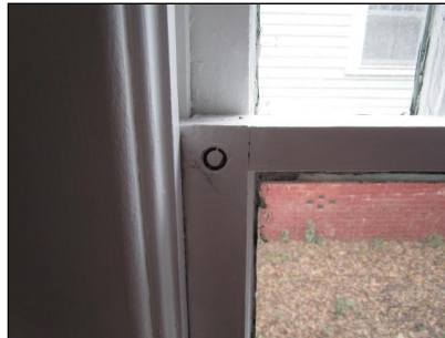
All main level windows were pinned shut.
