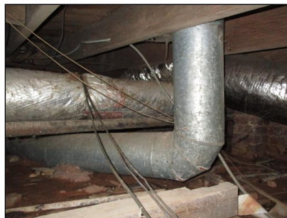
Add insulation where missing
