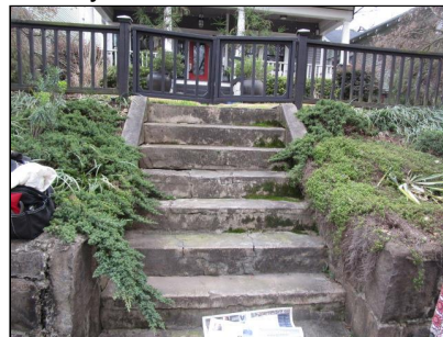
Add handrail to the stairs at the front of the house.
