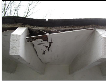
Damaged decking, leaking in the roof.
