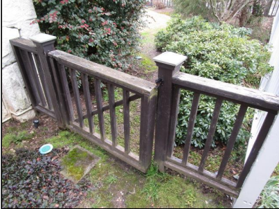
Gates do not close and latch properly
