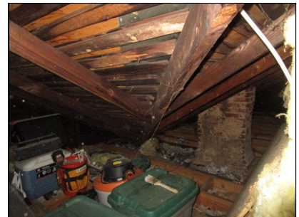
Add a purlin and brace system to prevent sagging of the roof.
