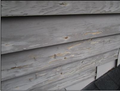
Paint weathered and peeling on the siding
