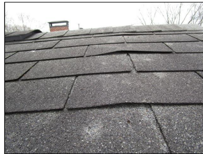
Nail pops lifting shingles in several places.
