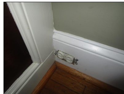
Add missing cover plates on the main level
