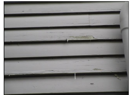
Paint weathered and peeling on the siding
