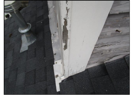
Paint on the trim weathered and peeling
