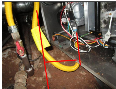
Flex line not permitted through furnace wall, sediment trap missing.
