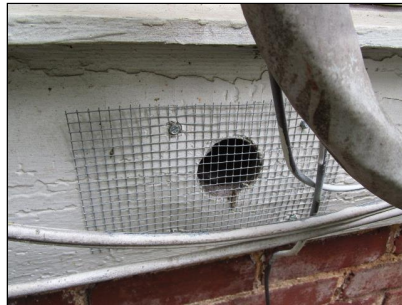
Have holes in the siding repaired.
