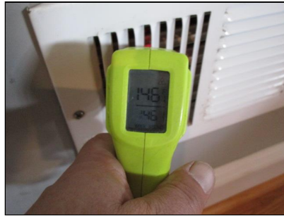
Regular heat tested and functional.
