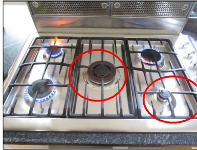
Burners did not light, were lit by hand.
