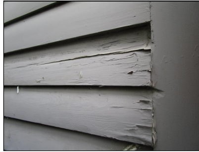
Replace damaged siding
