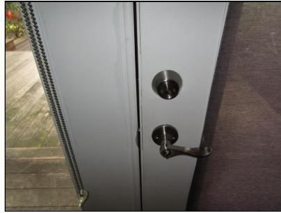
Rear doors stick at the bottom and do not latch properly.
