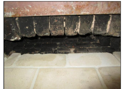
Add dampers where missing
