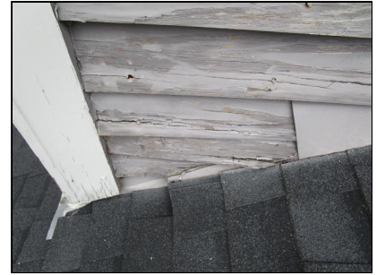
Replace damaged siding
