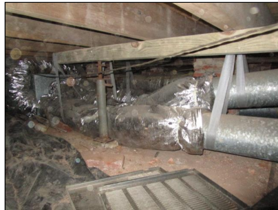
Remove ducts from ground contact.
