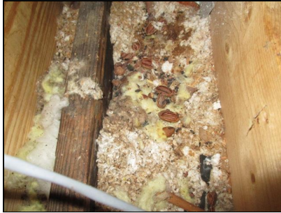
Signs of rodent intrusion in the attic and crawlspace.
