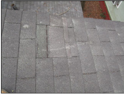
Soft area indicates leak at the upper right rear of the roof.
