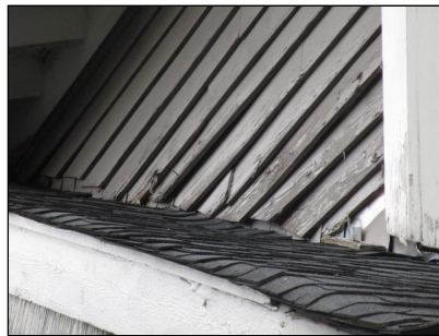
Replace all damaged siding.
