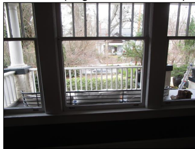
Many windows painted shut.
