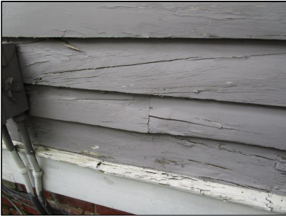
Replace damaged siding
