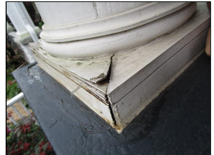
Repair all damaged trim
