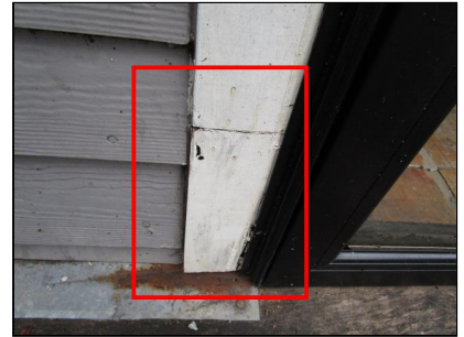
Repair all damaged trim
