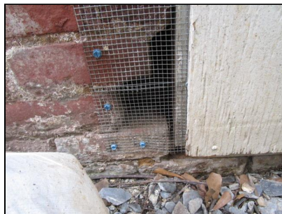
Replace the missing bricks at the crawlspace entry door.
