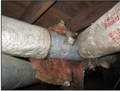
Add insulation to all ducts where damaged or missing
