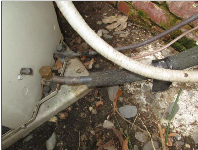
Add insulation where missing
