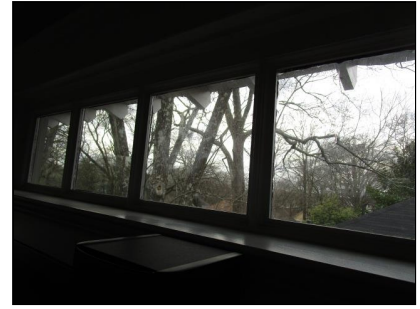
Failed windows in the upper master sitting area
