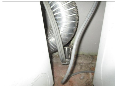
The dryer receptacle is loose from the wall.
