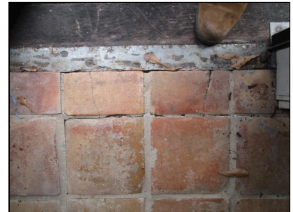
Tiles at the laundry entry door are cracked and loose.
