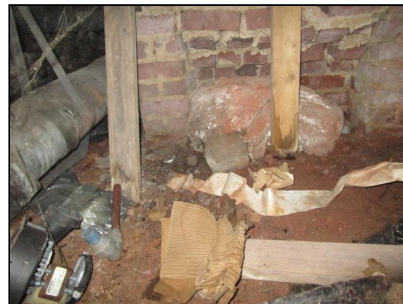
Support posts missing footers, in contact with the soil.
