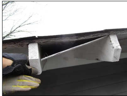
Damaged decking around perimeter of the roof.
