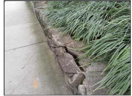
Extensive deterioration of the front retaining wall.
