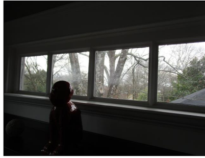
Failed windows in the upper master sitting area
