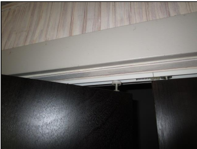
Laundry doors do not track properly
