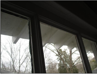
Replace cracked upper level window
