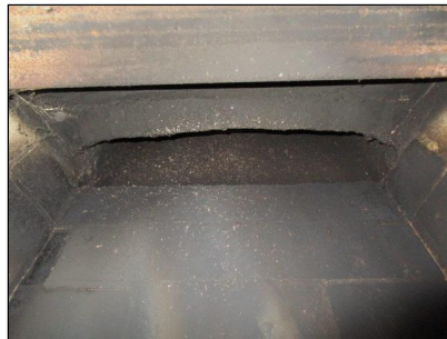
Have chimney swept and inspected, repaired as needed.
