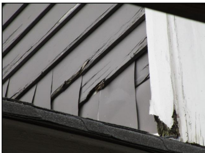
Replace all damaged siding.
