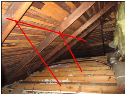
Add a purlin and brace system to prevent sagging of the roof.
