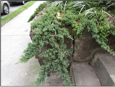
Cracks and settlement in the retaining wall.
