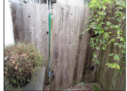
Repair or replace all gates to open and close properly
