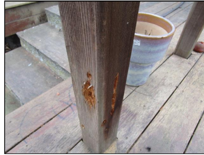
Repair carpenter bee damage to the posts.
