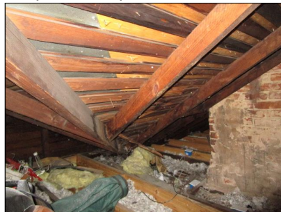
Add a purlin and brace system to prevent sagging of the roof.
