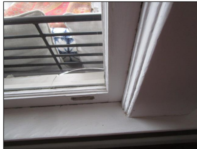
Replace all cracked window panes.
