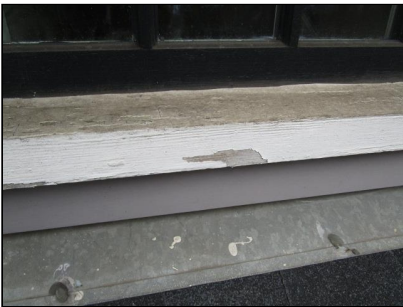
Paint weathered and peeling
