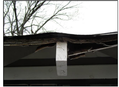
Damaged decking around perimeter of the roof.
