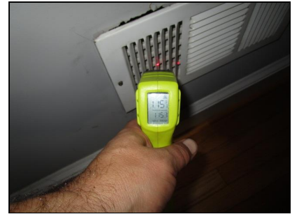
Emergency heat tested and functional.
