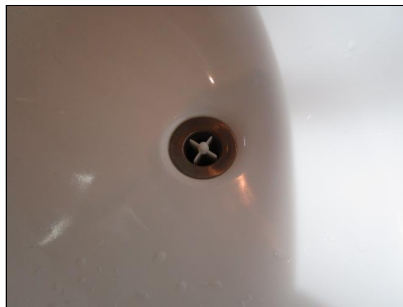
Replace the missing pop up drain.
