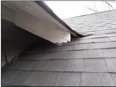
Repair all damaged trim
