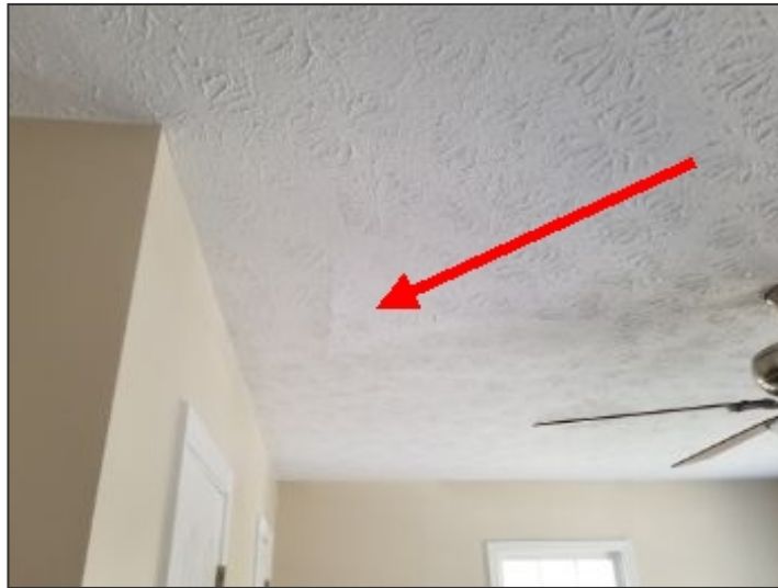
Water stain at master bedroom ceiling
