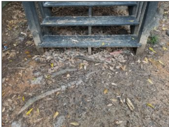
No landing and improper support of deck stairs
