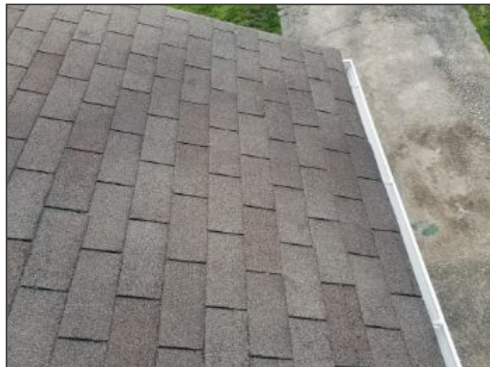
Normal wear and tear at shingle surfaces
