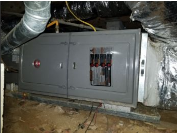
Furnace located in crawl space
