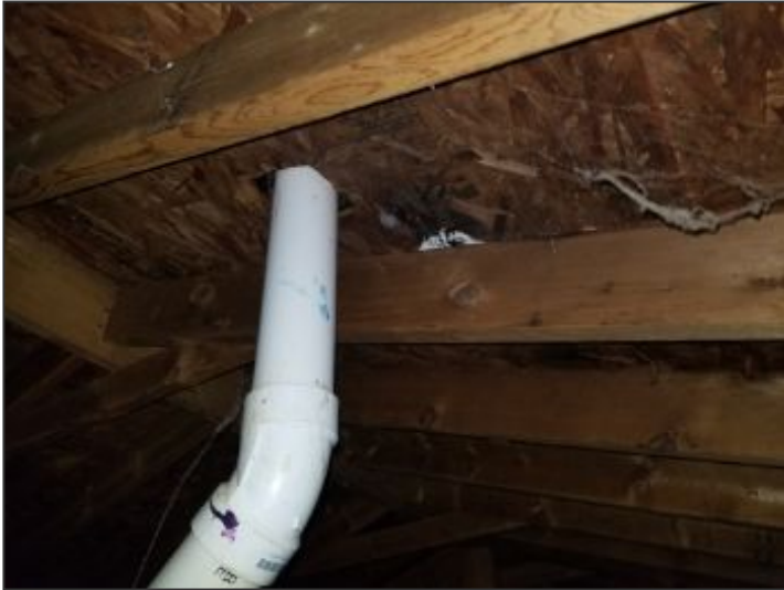
Evidence of a leak at center roof plumbing vent
