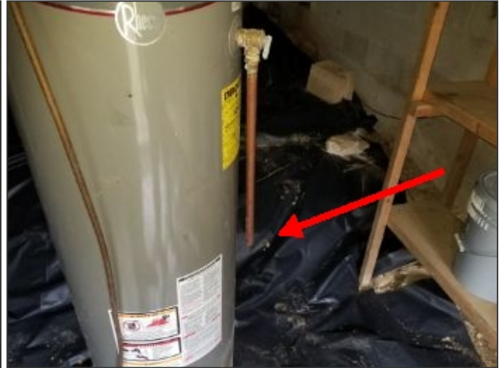
Temperature and pressure relief drain terminating into crawl space
