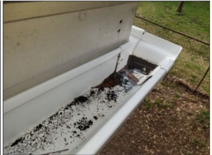
Rear corner gutter holding water
