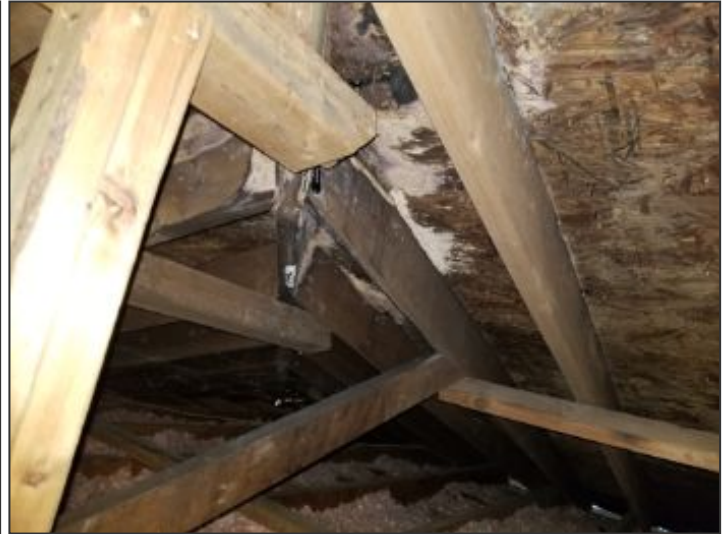
Evidence of a previous leak at right right roof ridge above master
