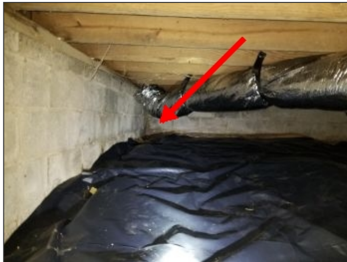
Evidence of previous water entry at front left foundation corner
