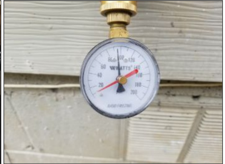
Water pressure too high at 95 PSI
