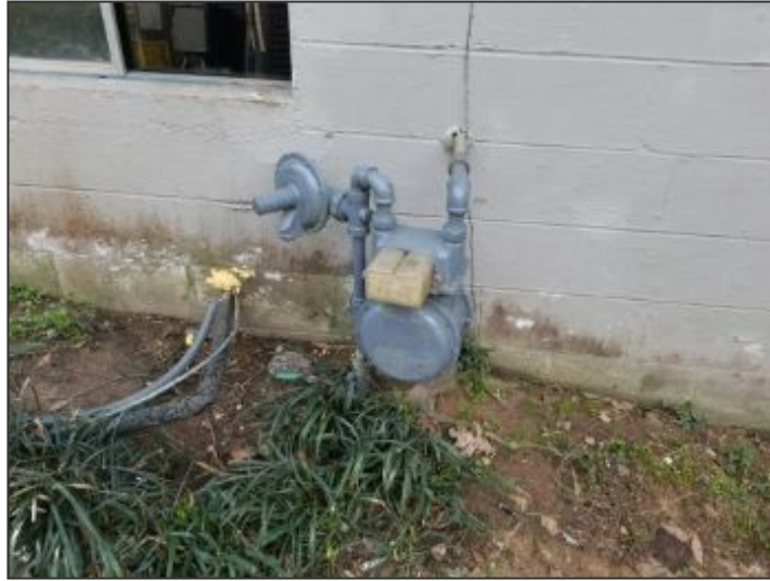
Gas meter at right side wall
