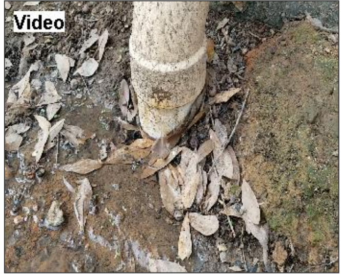
Active leak at rear exterior plumbing drain
