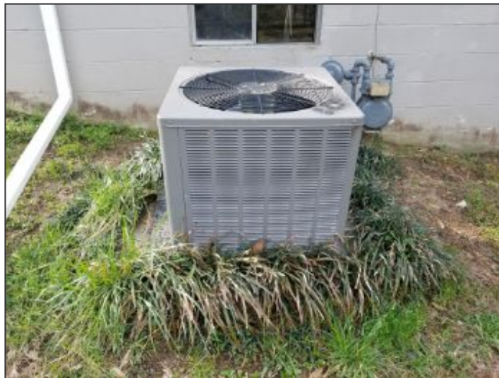
AC unit at right side wall
