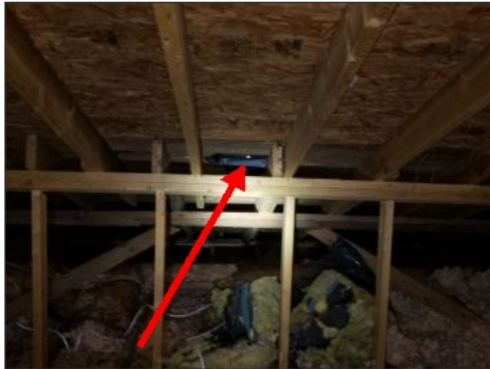
Missing roof decking with daylight through shingles at front roof
