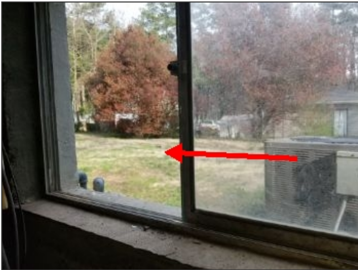
Unprofessionally repaired window in crawl space
