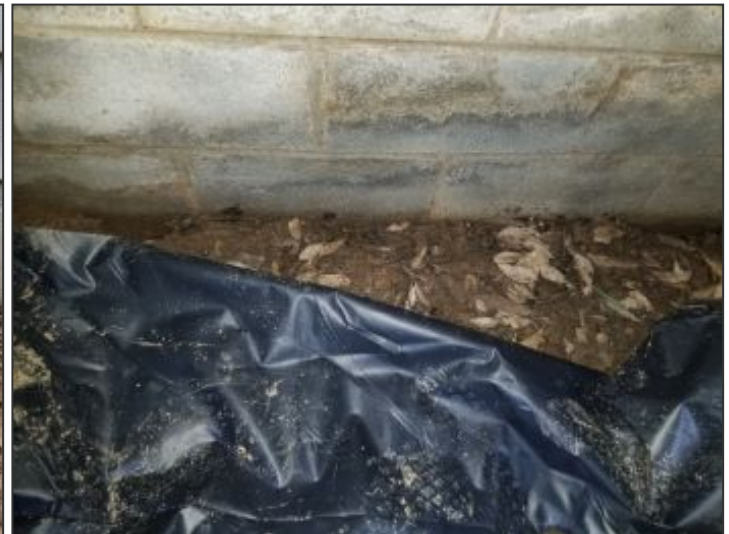
Wet conditions at rear foundation wall in rear crawl space
