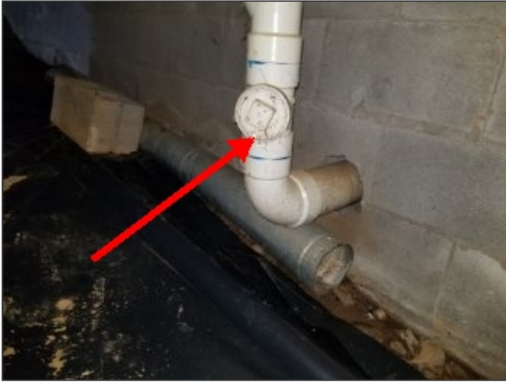
Active leak at plumbing drain clean out cap
