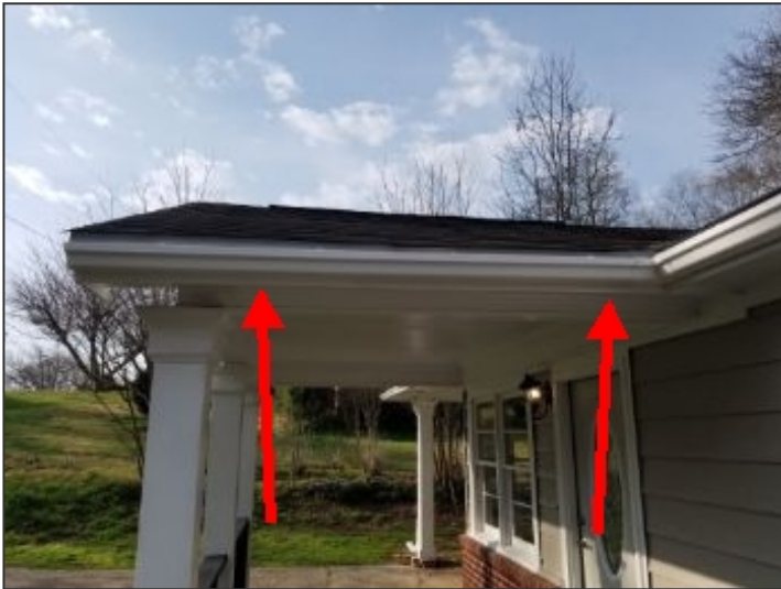
Improper gutter slope at right side porch roof
