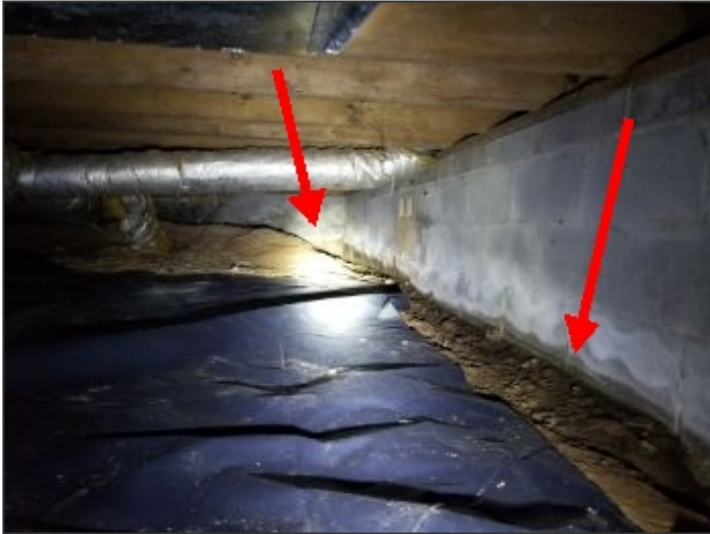
Evidence of water entry at rear and left corner foundation wall
