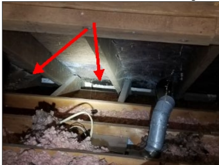
Evidence of roof leaks at rear roof
