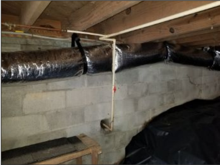
Main water cut-off handle located in crawl space
