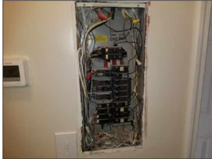
View inside main panel box
