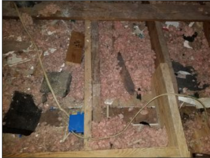
Poor insulation depth in attic
