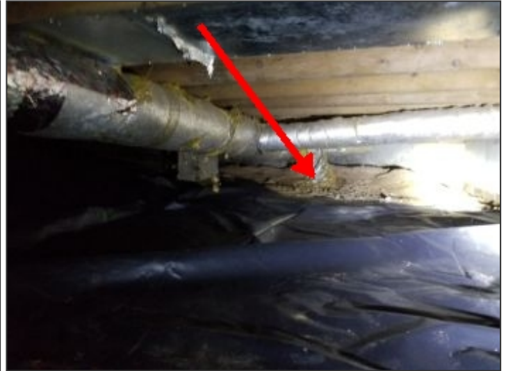
Missing vapor barrier below rear family room
