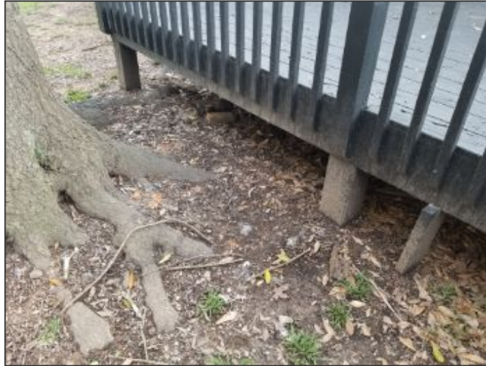
Wood posts below grade at rear deck
