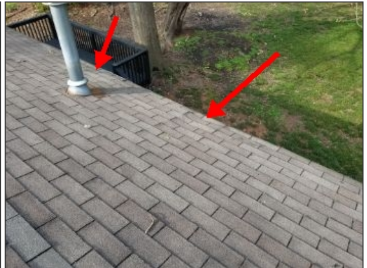
Sagging roof surface at rear
