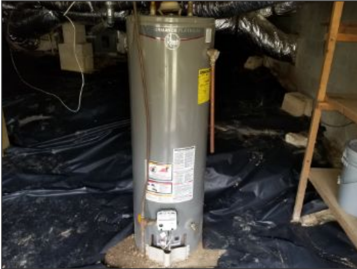
Water heater located in crawl space
