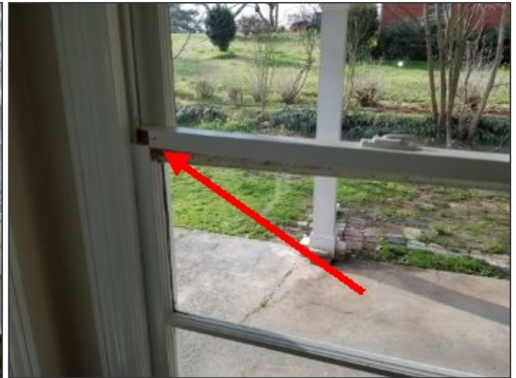
Damaged / loose window frame in front living room
