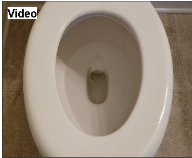
Toilets bubbling during testing of fixtures
