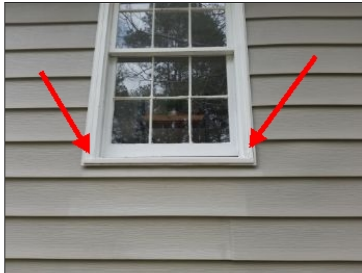
Damaged wood trim at rear master bedroom window
