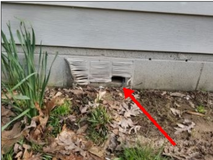
Damaged foundation vent at left side wall
