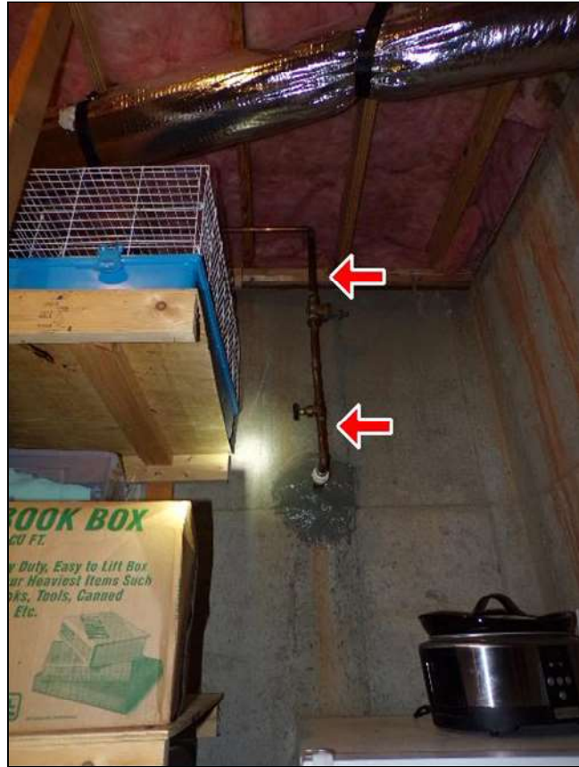
7.2 Missing bonding wire - main shut off
