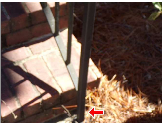
1.0 Handrail newel post is not attached properly.
