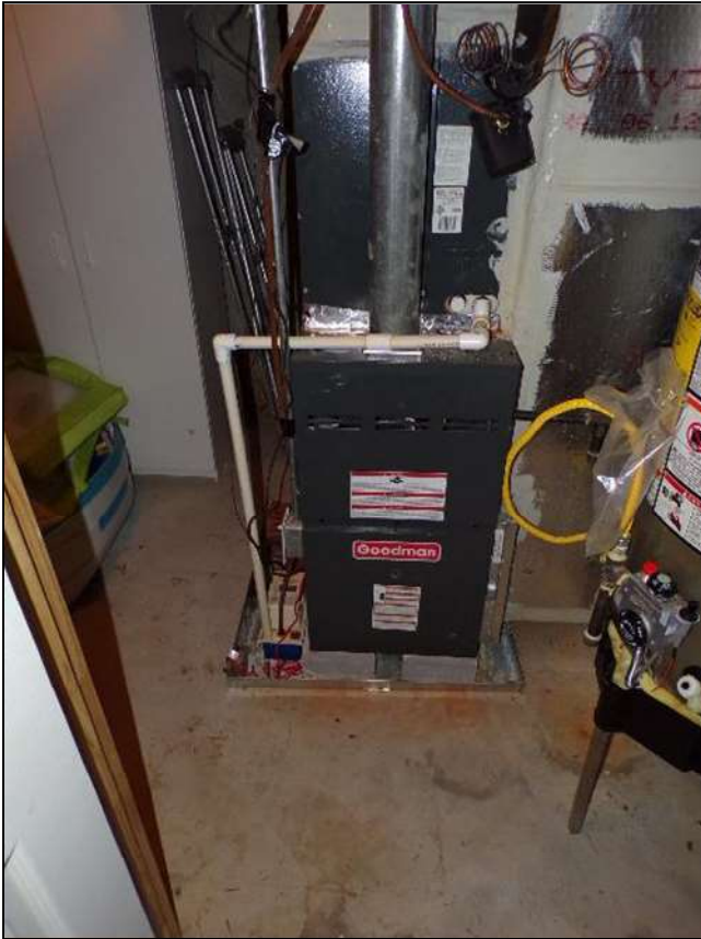
9.0 Basement unit - Goodman
