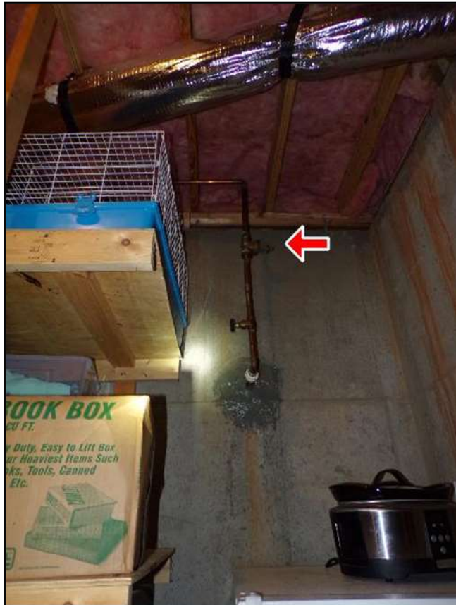
7.2 PRV - Pressure reducing valve
