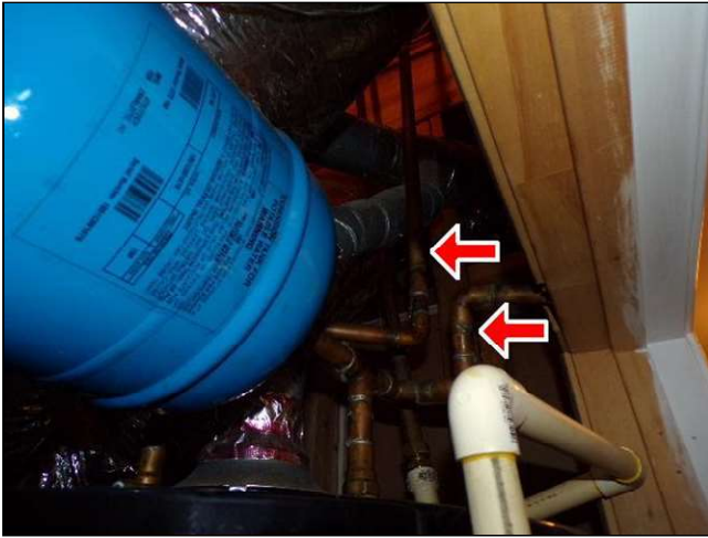
7.2 Missing bonding wire - water heater
