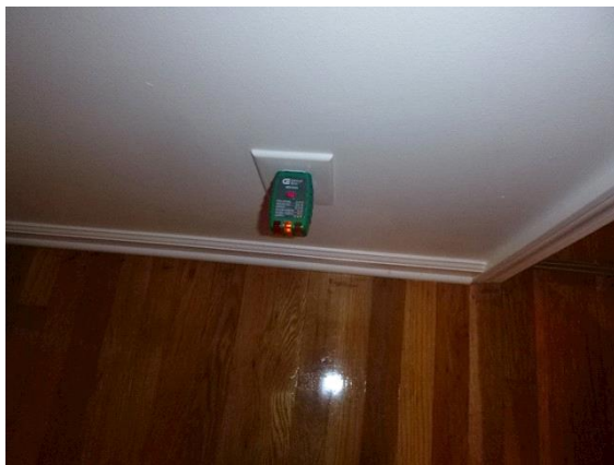
outlet not grounded - example
