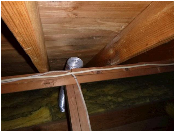
Attic Ventilation: Bathroom venting into attic
