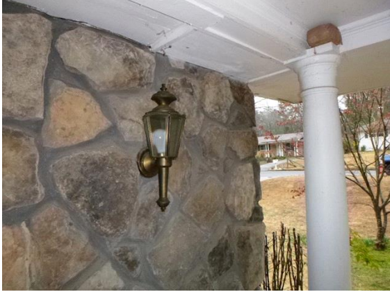
Exterior Surface: light not working
