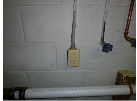
Laundry Facilities: outlet not GFCI
