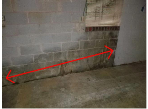
Interior Foundation: Signs of water intrusion
