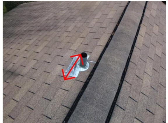
Roofing: sealant on nails is deteriorated/missing
