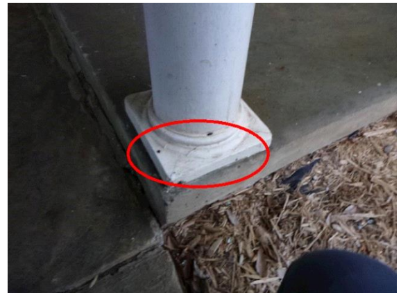
Porches / Stoops: wood rot
