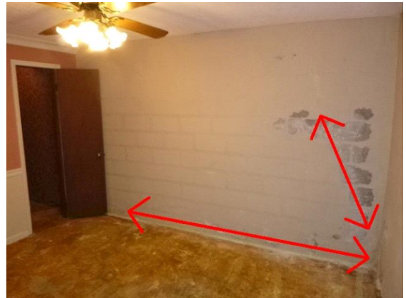
Interior Foundation: efflorescence
