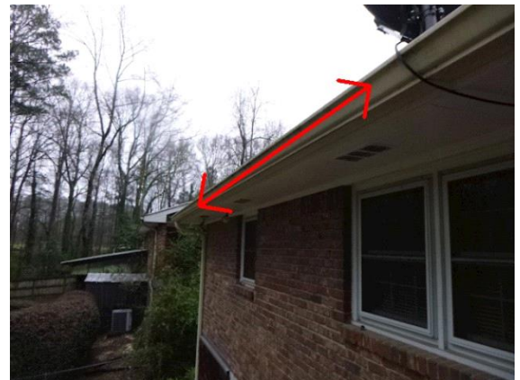
Gutters/Down Spouts: signs of overflowing
