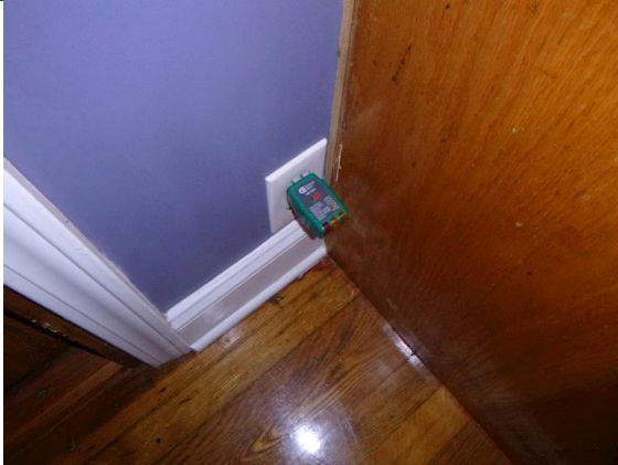
Electrical: outlet not grounded - example
