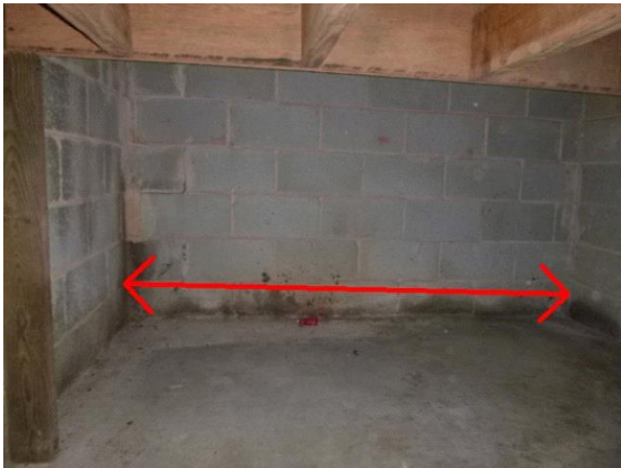
Interior Foundation: efflorescence
