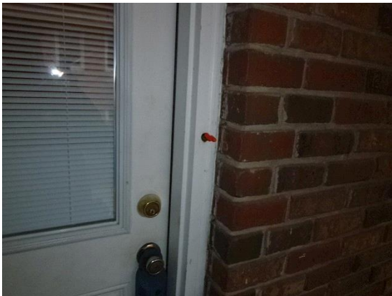
Exterior Doors: missing doorbell
