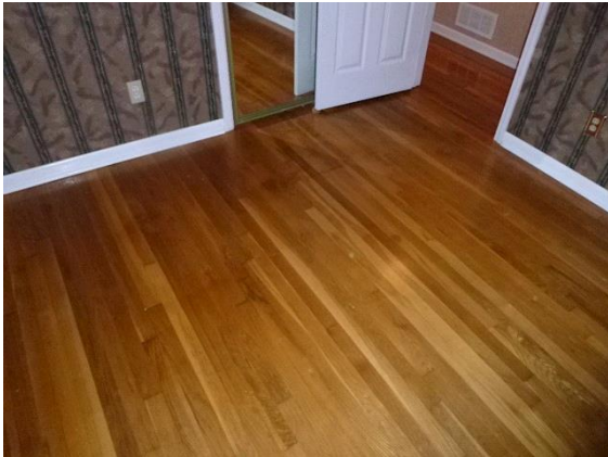
Floor/Slab: creaking flooring
