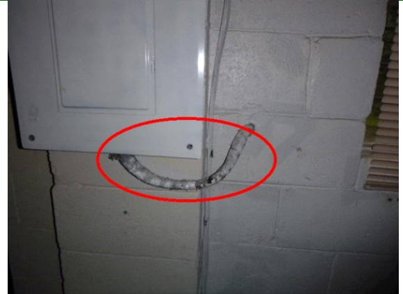
Electrical: deteriorated sheathing
