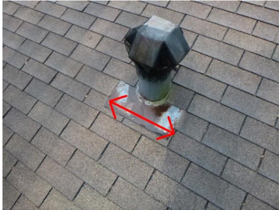
sealant on nails is deteriorated/missing
