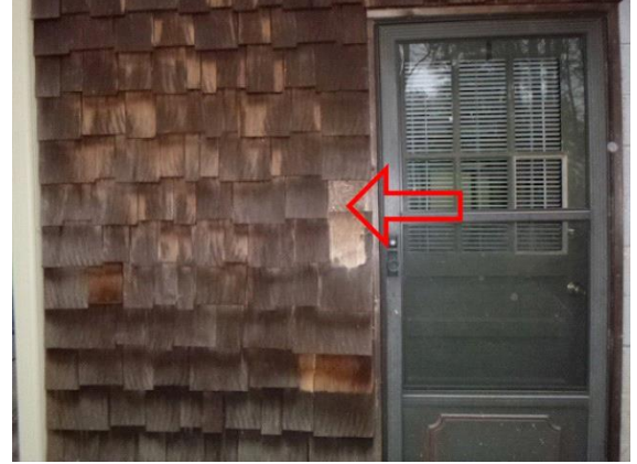
Exterior Surface: missing siding
