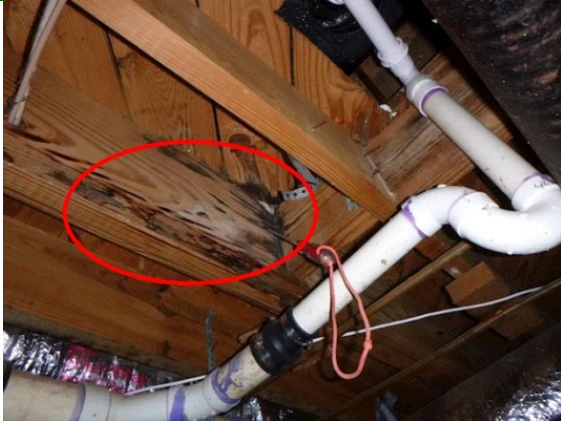
Under Floor Framing & Support: wood rot, Suspected fungal growth
