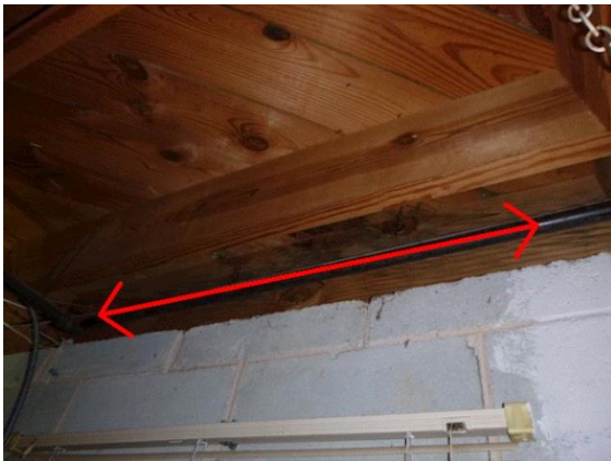
Under Floor Framing & Support: Suspected fungal growth
