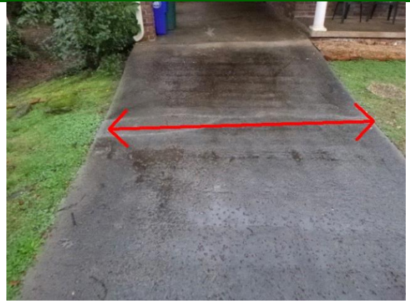
Driveway: Repair cracking
