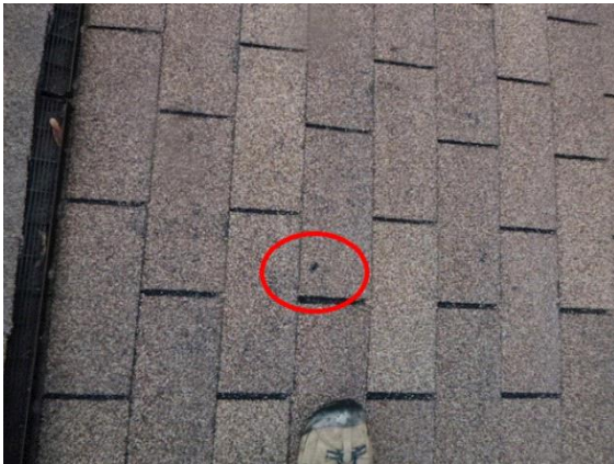
Roofing: damaged shingle, active leak
