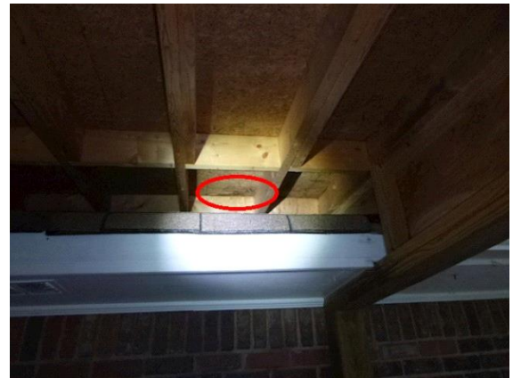
Roofing: leaking above deck
