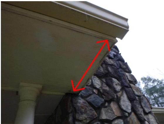
Exterior Surface: wood rot
