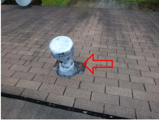
Roofing: sealant on nails is deteriorated/missing
