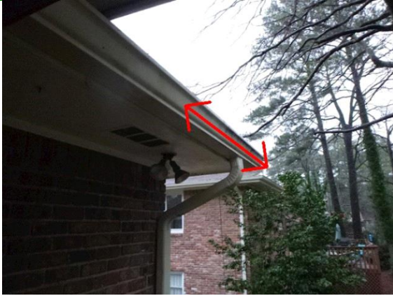
Gutters/Down Spouts: signs of overflowing
