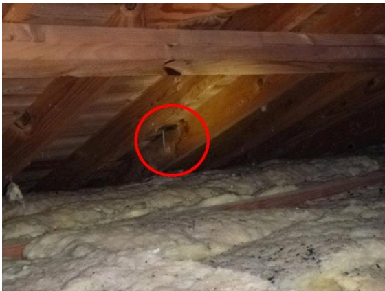
Attic Framing/Sheathing: Water stains
