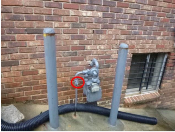
Plumbing: Gas shutoff valve
