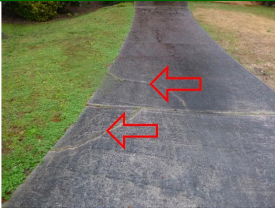
Driveway: Repair cracking
