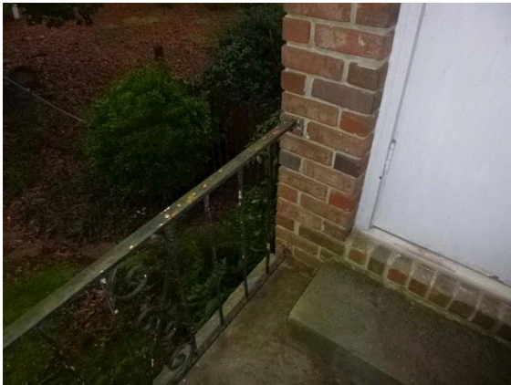
Garage/Carport: loose railing, balusters spaced at 6"
