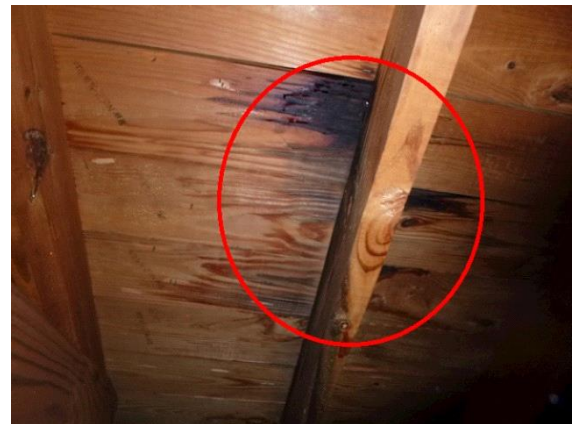
Attic Framing/Sheathing: Water staining, active leak
