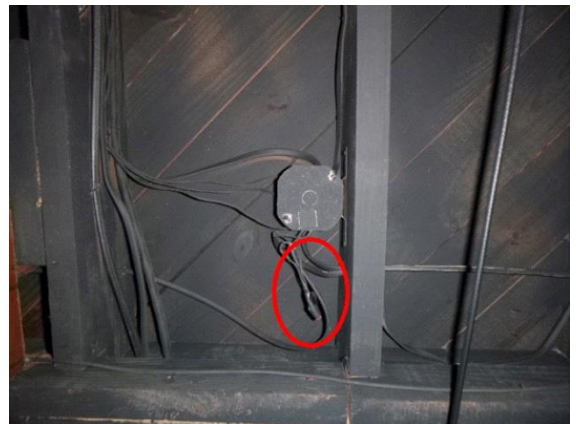
Electrical: exposed splice
