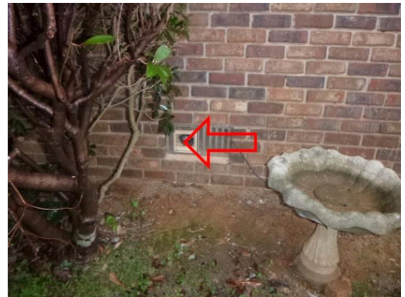
Exterior Surface: damaged vent
