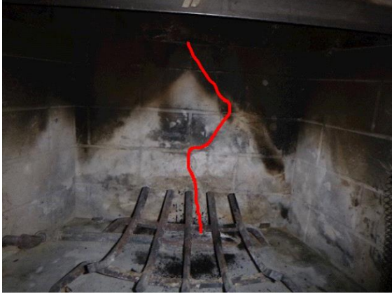
Fireplace/Stove: Damaged firebox
