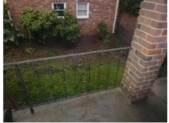
Garage/Carport: loose railing, balusters spaced at 6"
