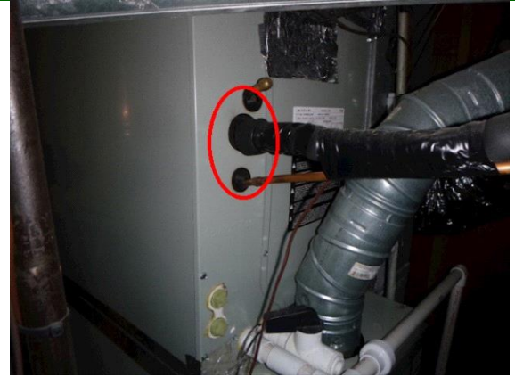
Heating #1: seal cabinet
