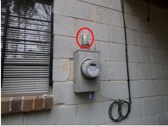
Electrical: frayed cable sheathing
