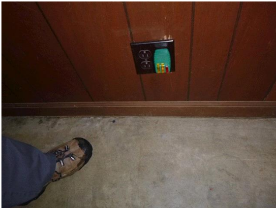
Electrical: outlet not grounded - example
