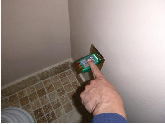
1/2 Bathroom: Outlet not GFCI protected
