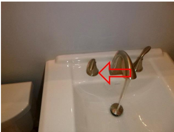
Hall Bathroom : loose handle
