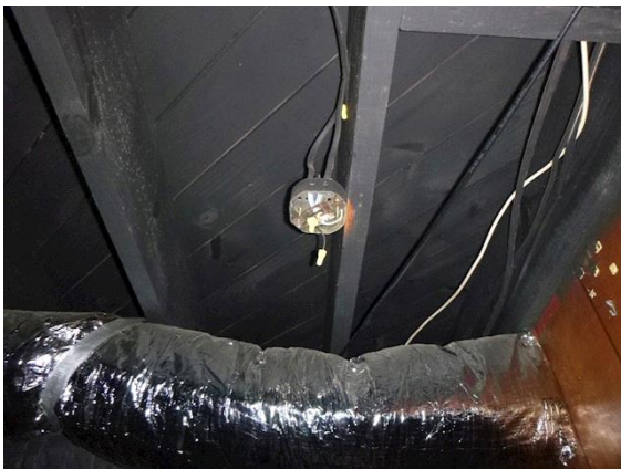
Electrical: open junction box
