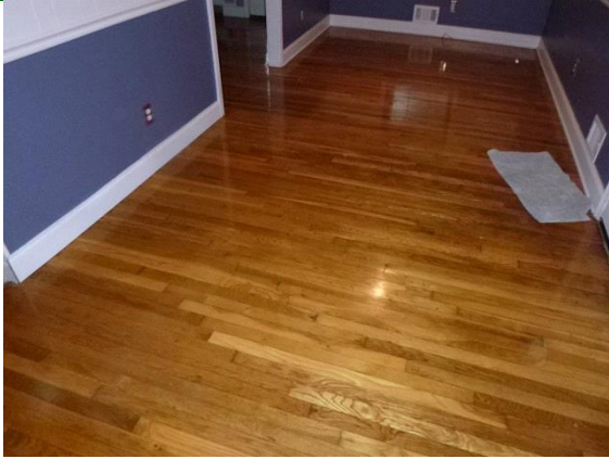
Floor/Slab: creaking flooring
