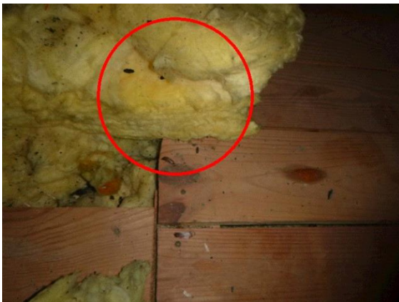
Attic Insulation: droppings
