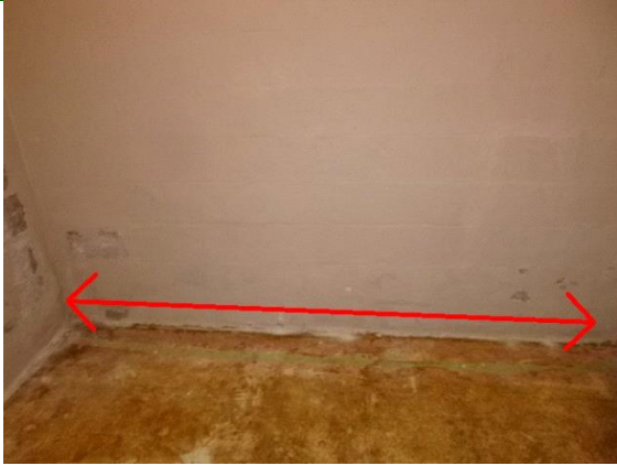
Interior Foundation: efflorescence
