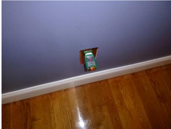
outlet not grounded - example
