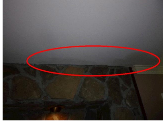
Family Room: water stains
