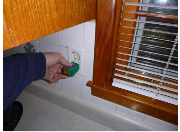
Kitchen: Outlet not GFCI protected
