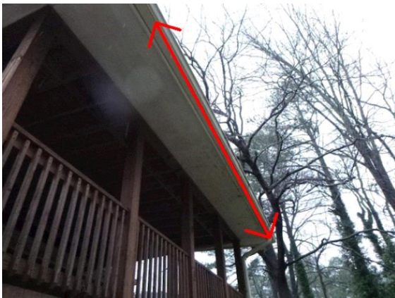
Gutters/Down Spouts: signs of overflowing
