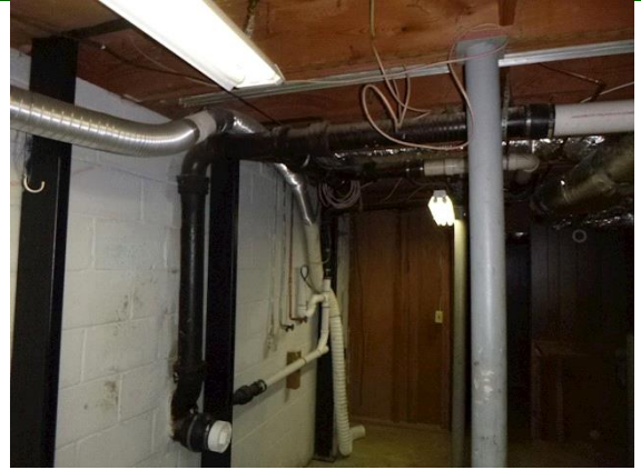
Plumbing: Cast Iron Drains
