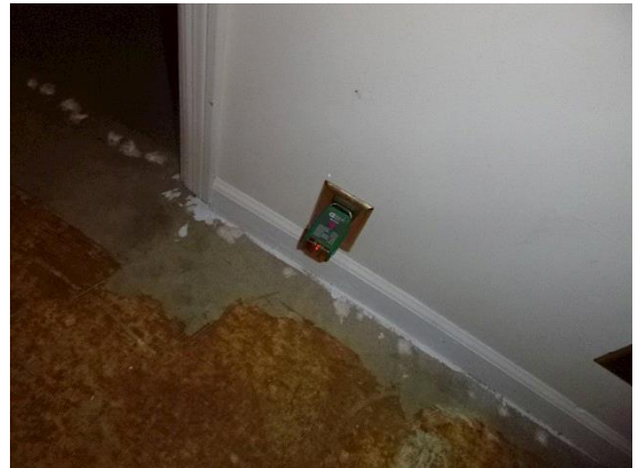
Electrical: outlet not grounded - example
