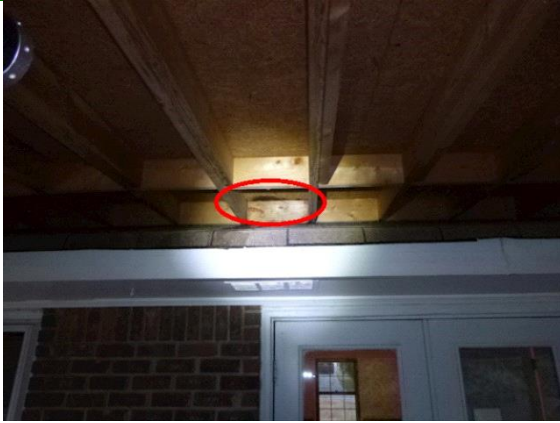
Roofing: leaking above deck
