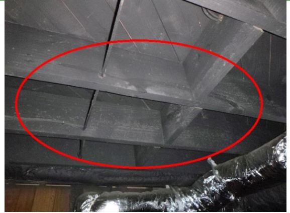
Under Floor Framing & Support: Suspected fungal growth
