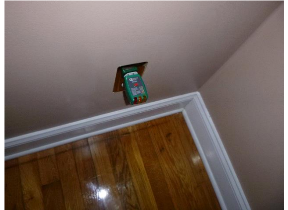
outlet not grounded - example
