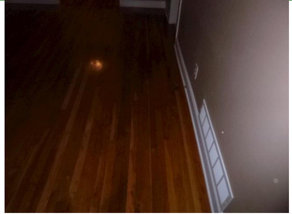
Floor/Slab: creaking flooring
