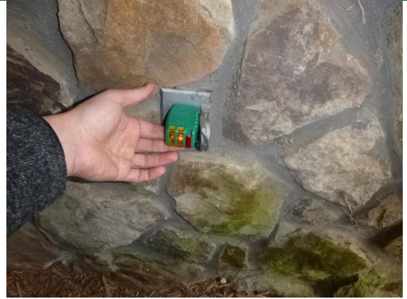
Exterior Surface: Outlet not GFCI protected or grounded
