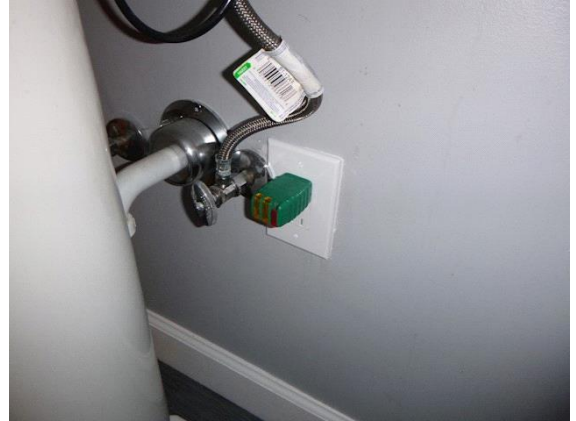
Hall Bathroom : no power
