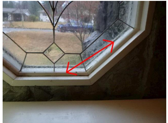
Family Room: cracked glass
