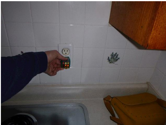
Kitchen: Outlet not GFCI protected
