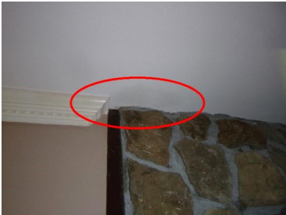
Family Room: water stains
