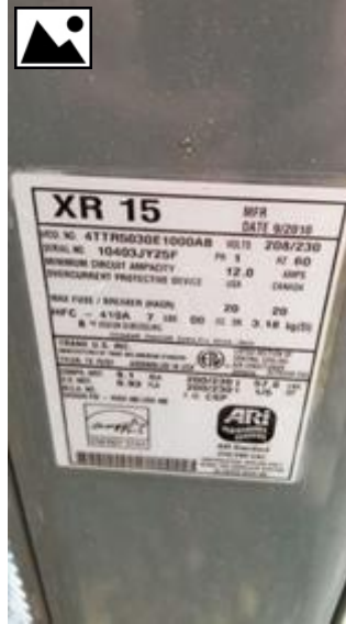
HVAC - Cooling System 3 Data Tag
