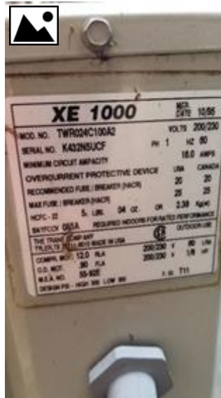
HVAC - Cooling System 1 Data Tag
