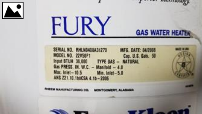
Plumbing - Water Heater 1 Data Tag
