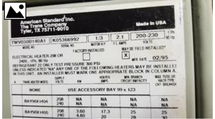
HVAC - Heating System 3 Data Tag
