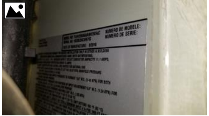
HVAC - Heating System 1 Data Tag
