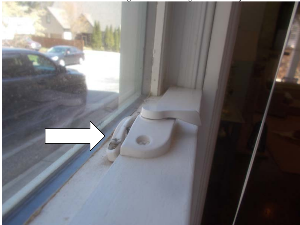
Window locks are coming loose in the rear hallway
