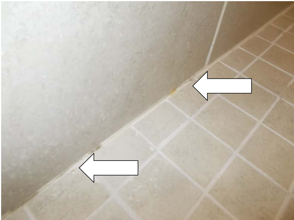
Caulking needed in the master bathroom shower
