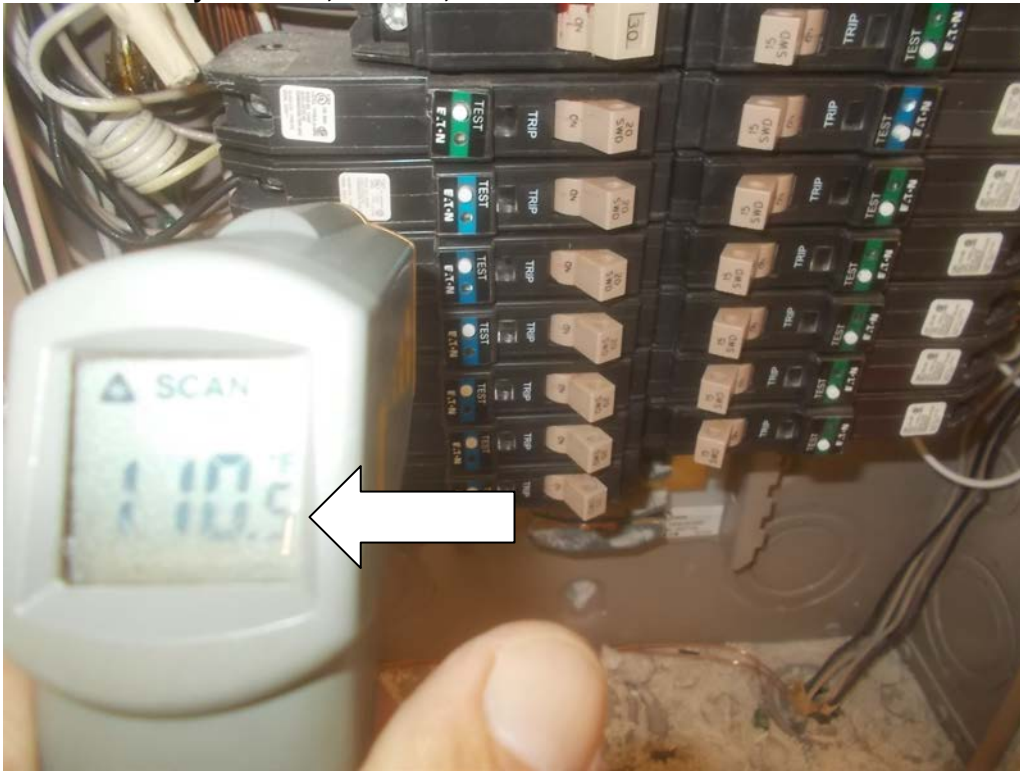
ARC fault breakers are 110 degrees
