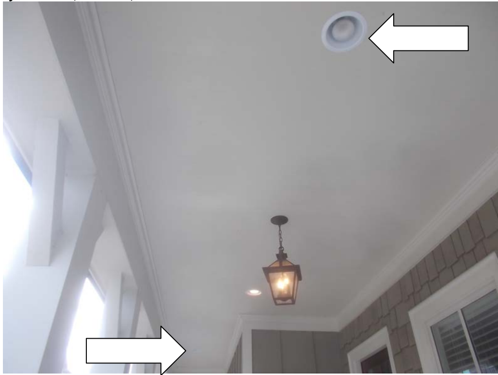
Can lights on the front porch are not working
