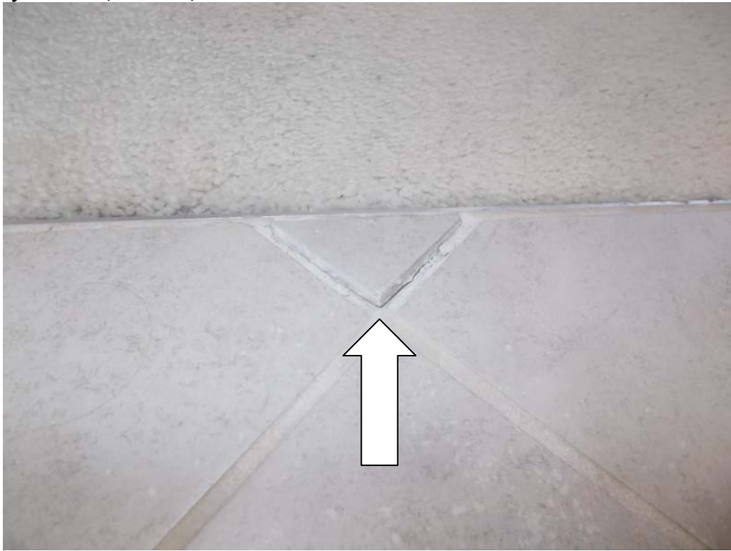
Small loose tile in front of the master bathroom door
