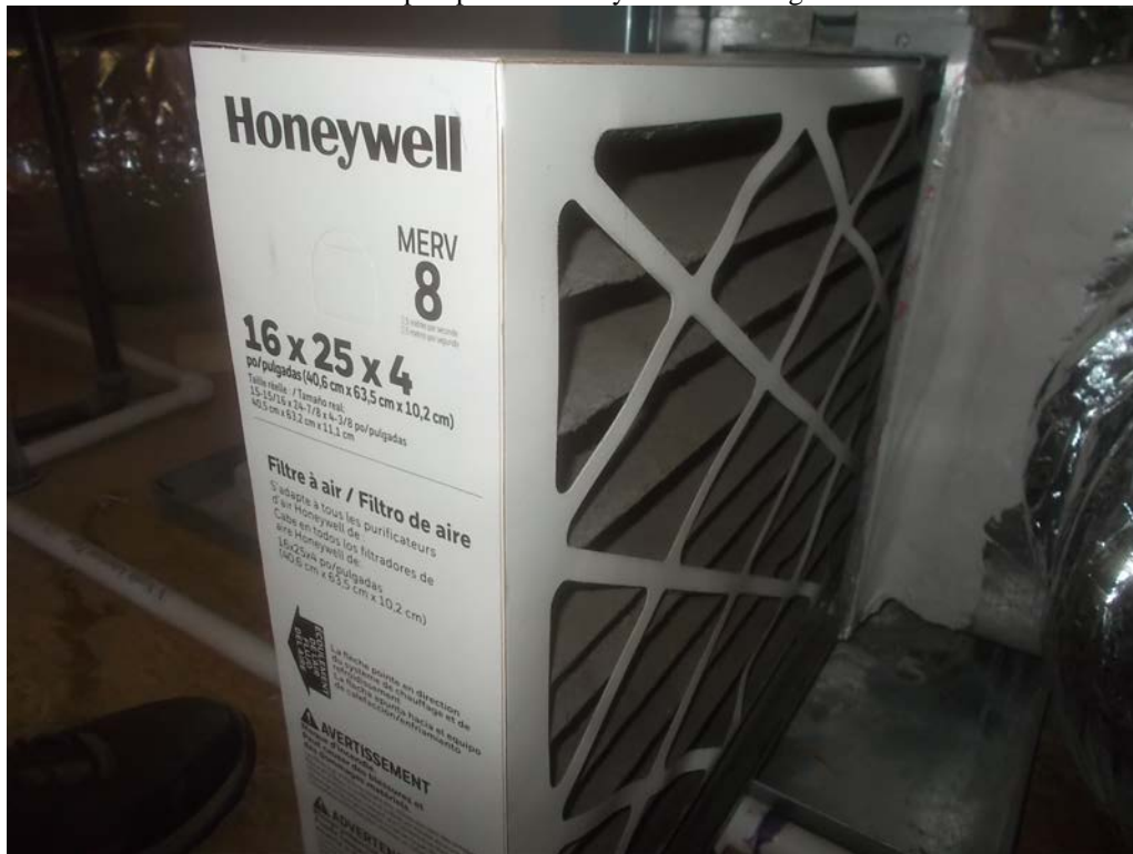
The furnace air filter is dirty and needs to be replaced
