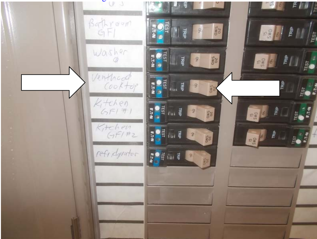
ARC fault breaker for the vent hood cooktop does not trip when tested
