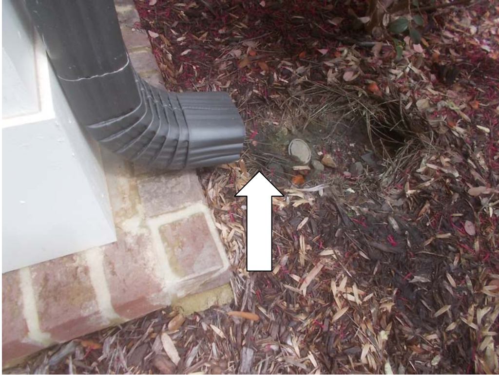
Downspout at the left front corner of the home needs to be extended away from the porch slab
