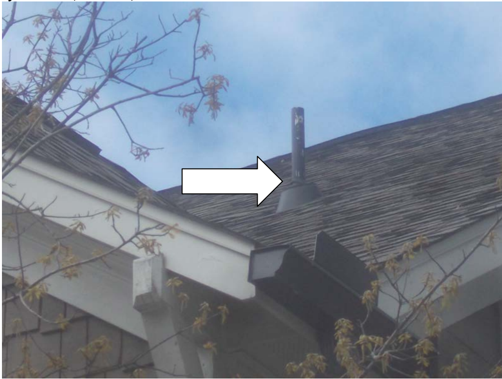
Boot on the front of the roof is torn
